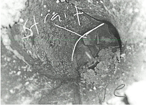
Figure 1. Damaged wye on city sewer main. Source: Subterranean Sewer Experts
