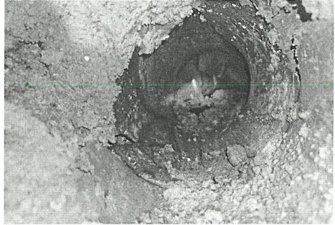
Figure 2. City sewer main wye cracked and collapsed. Source: Subterranean Sewer Experts
