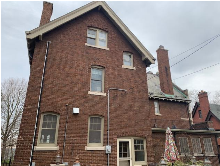
Rear door to be replaced.
