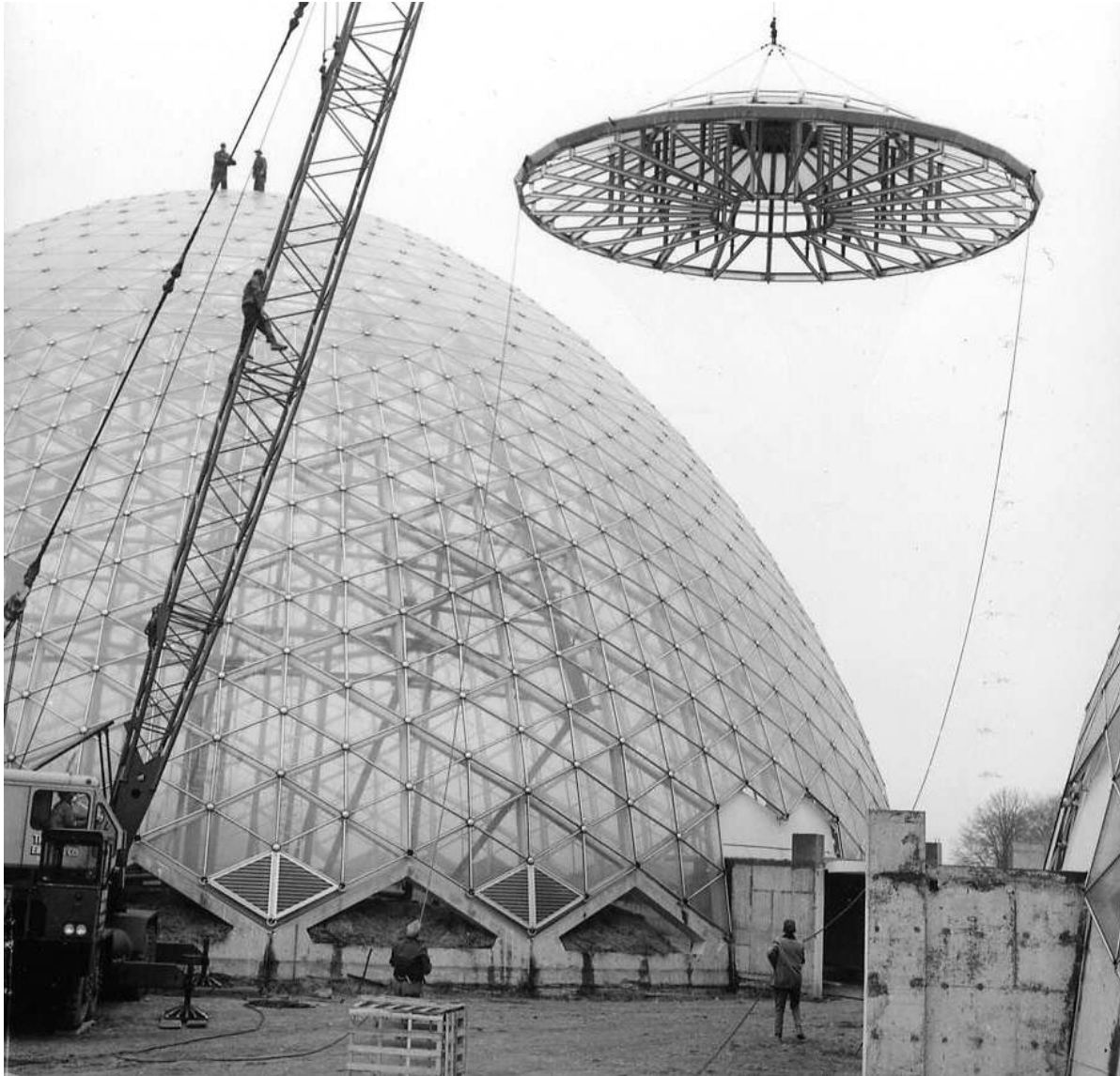
Figure 9. Photograph of the apex installation at the top of a dome. Source: Milwaukee County Parks Historic Photograph Collection.
