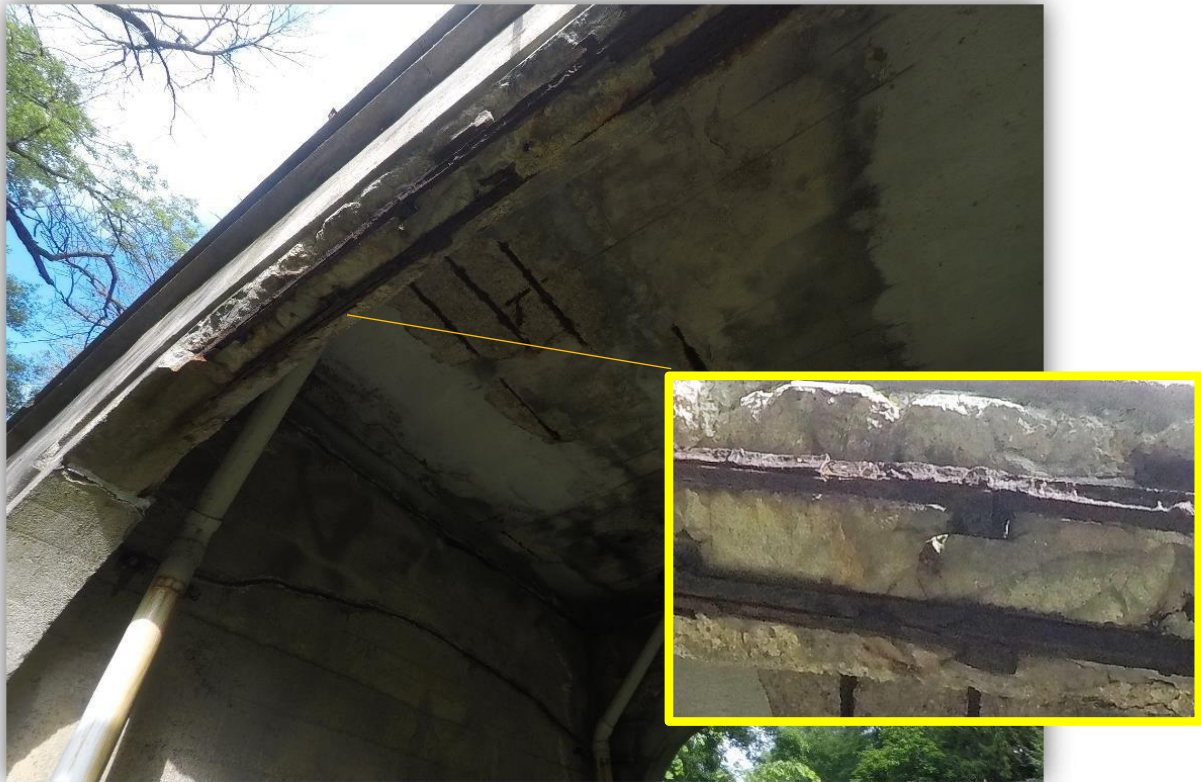
Corroded Kahn bars in the spandrel beam over the southeast tear drop piercing.
