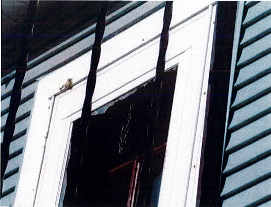
19-Front Elevation Storm door damaged
