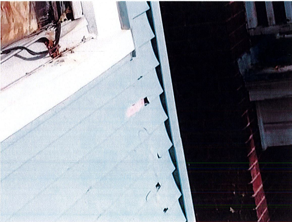
16-Front Elevation Siding damaged
