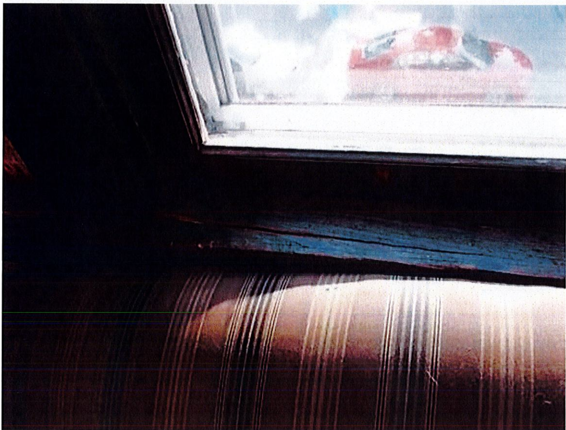
32-Living Room Window sill cracked
