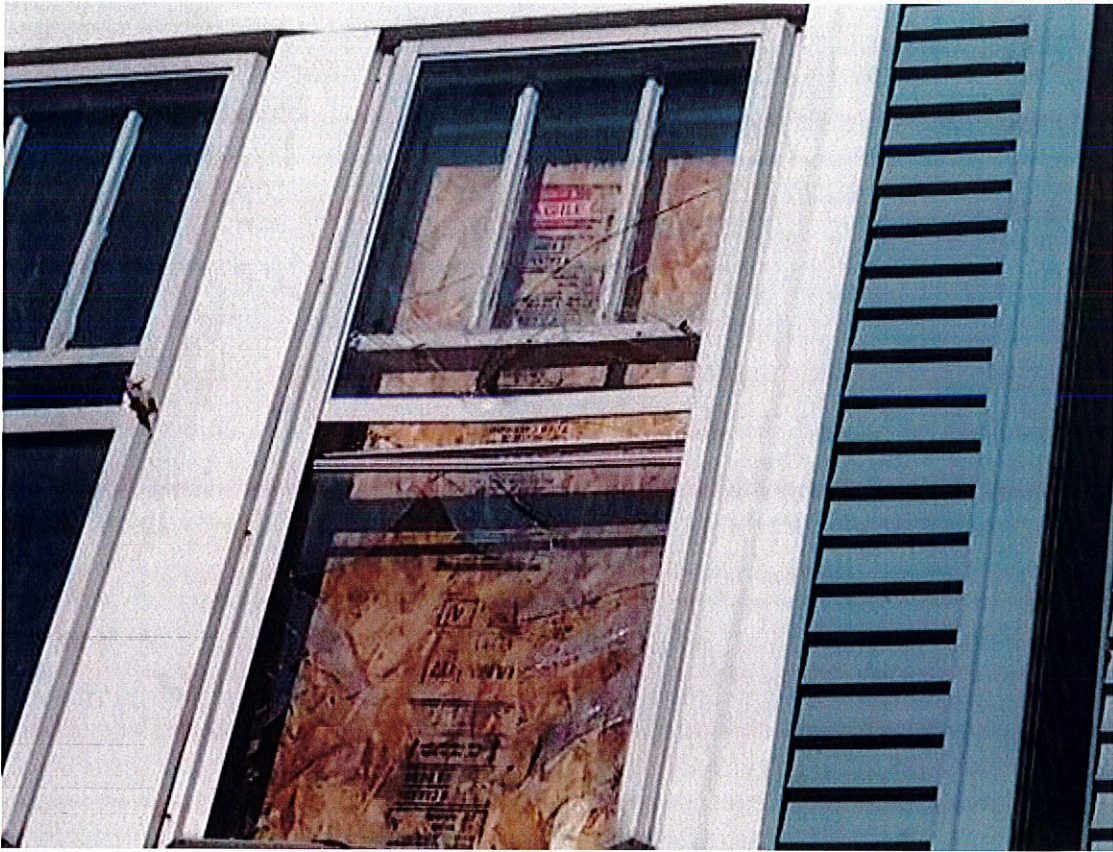
25-Front Elevation Damaged wood shales
