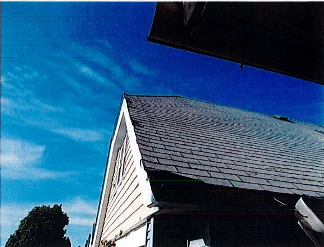
14-Right Elevation Shingles damaged
