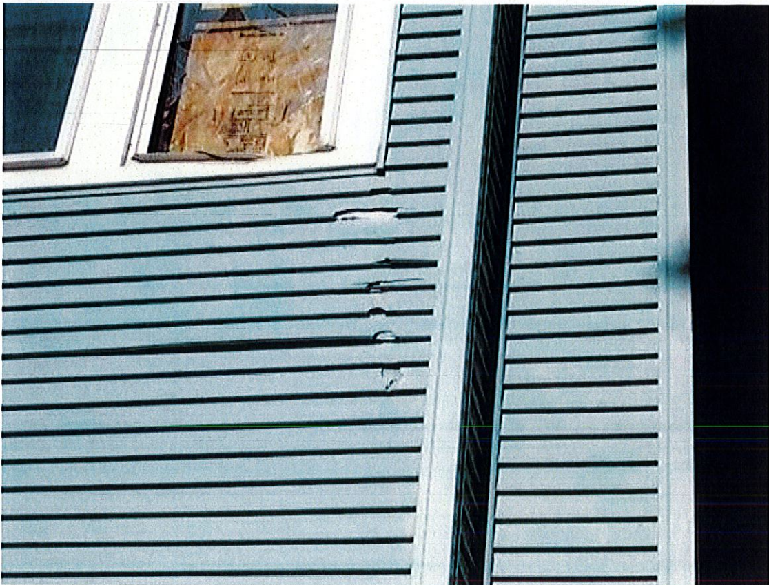
24-Front Elevation Siding damaged
