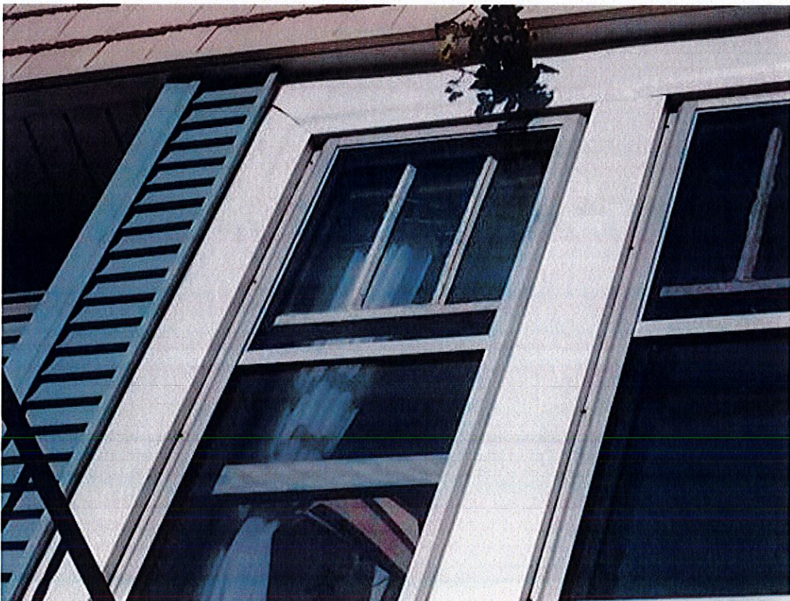
20-Front Elevation Storm windows damaged and window wrap
