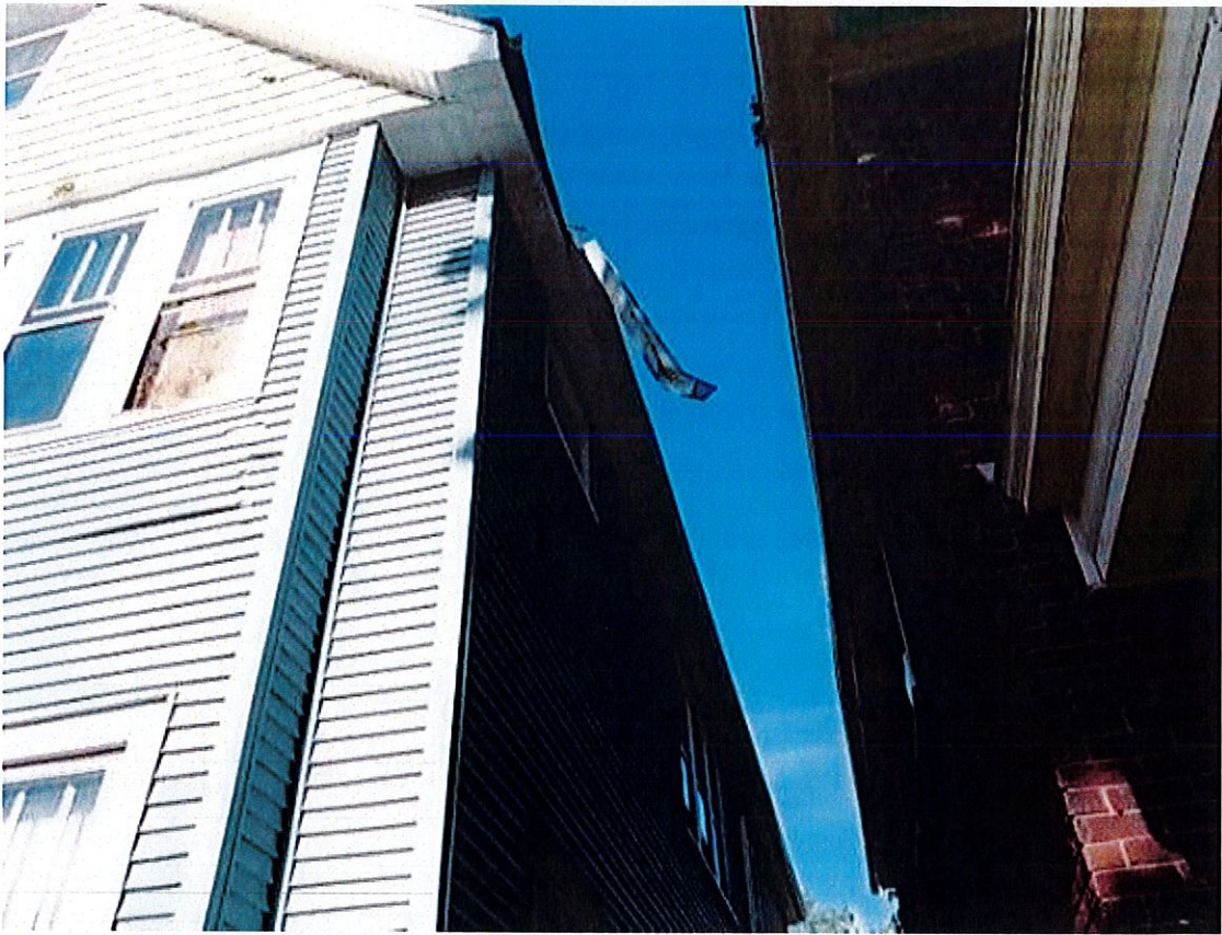
5-Risk Right Elevation gutter damaged
