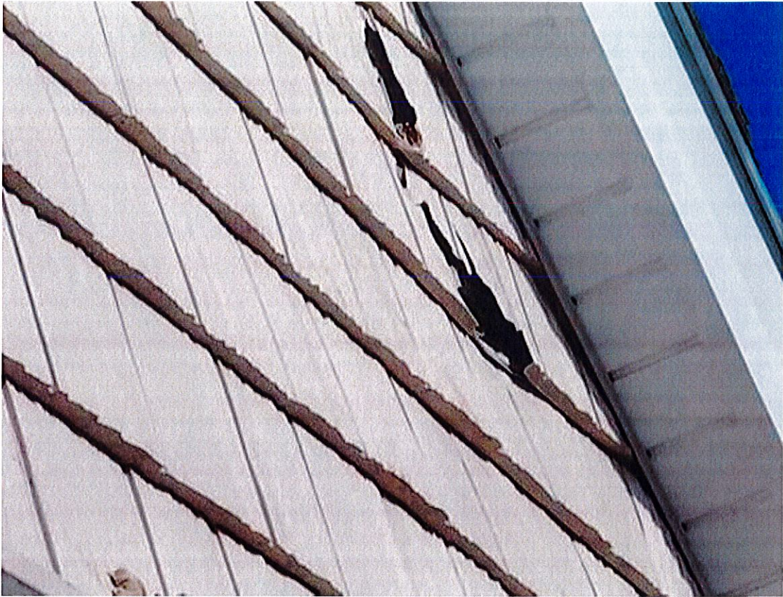
17-Front Elevation Metal shake Siding damaged
