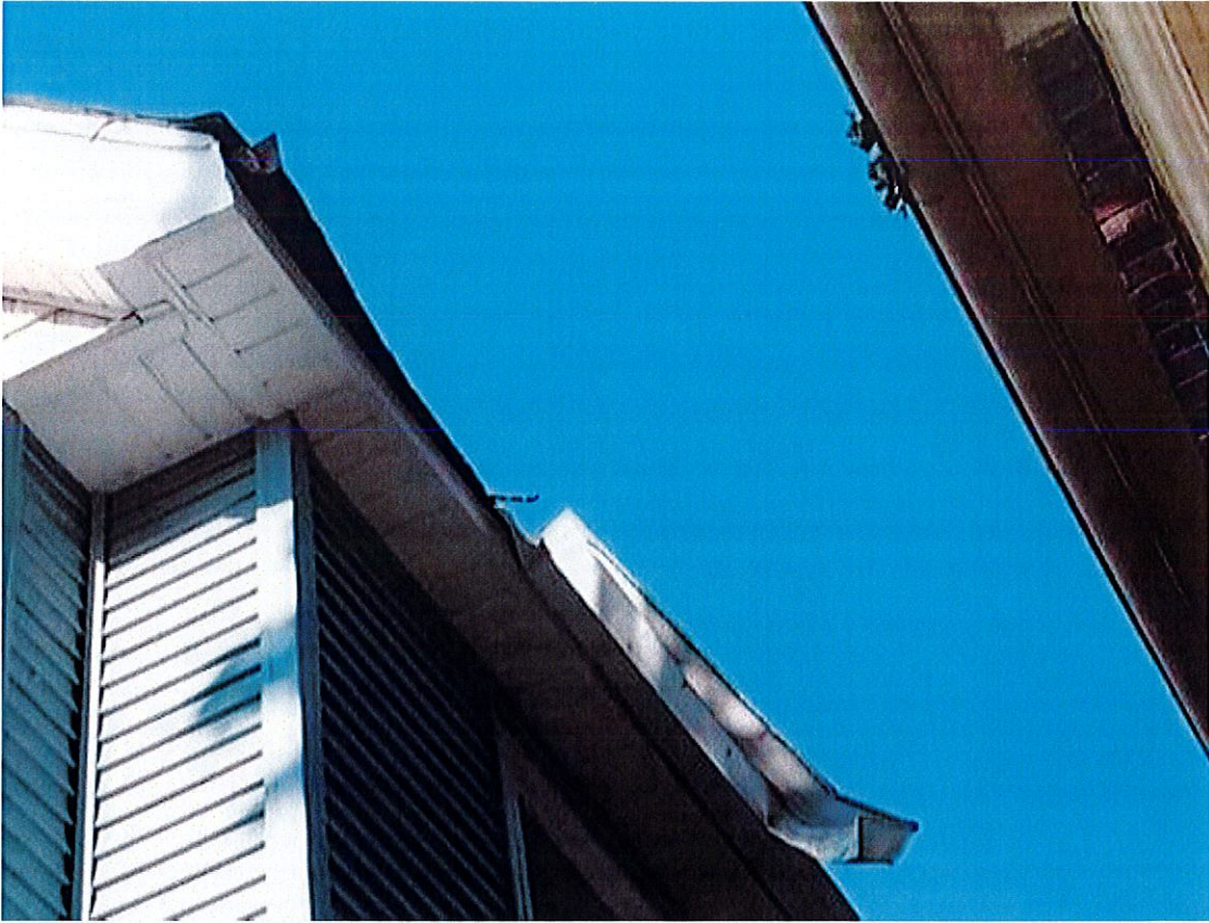
13-Right Elevation Gutter damaged
