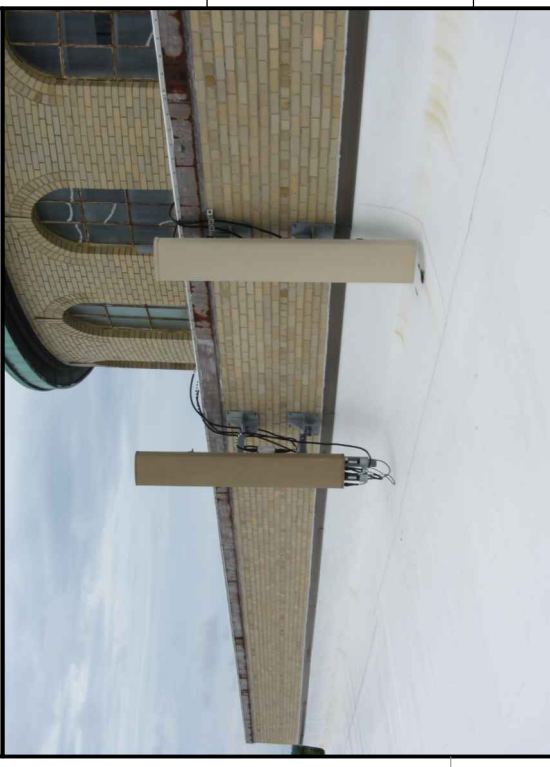
EXISTING T-MOBILE ANTENNAS - BETA SECTOR -
