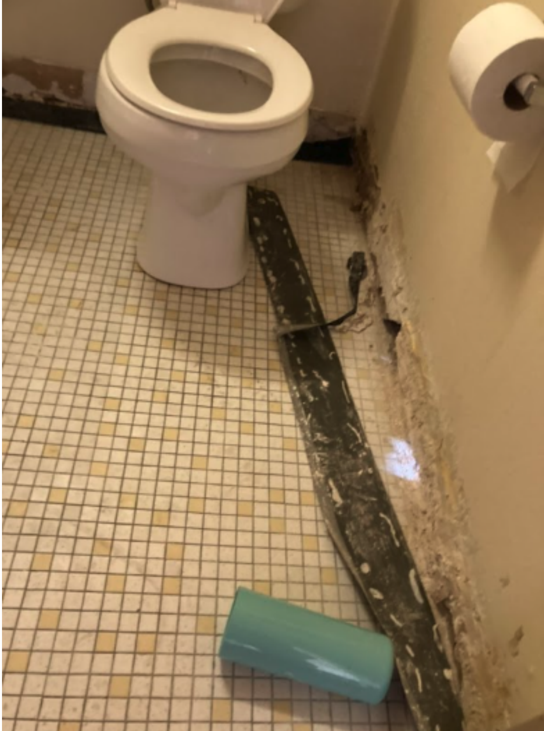
Description: Debra McQueen's bathroom at College Court. Her baseboards are busted and moldy. It smells terrible in her apartment.
