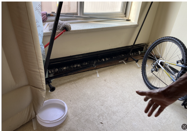
Description: Debra McQueen's bedroom at College Court. Her bedroom is uninhabitable, smelly, and in disrepair. She sleeps in her living room. She has reported these issues for years. She continues to pay full rent.
