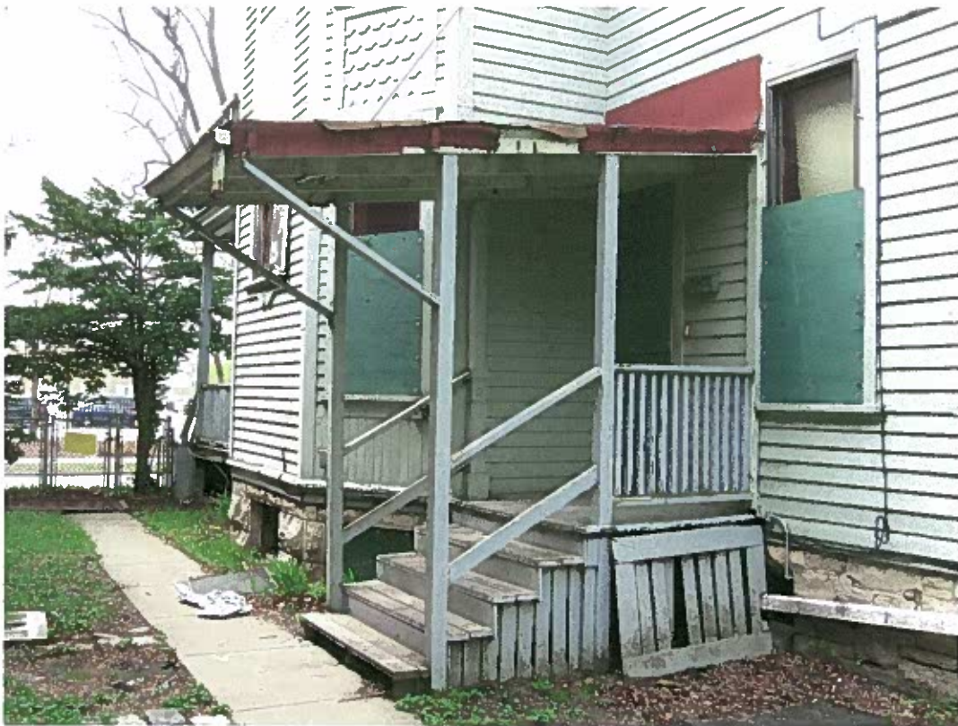
9. Side porch (North-East Elevation) with loss skirt and deteriorated roof
