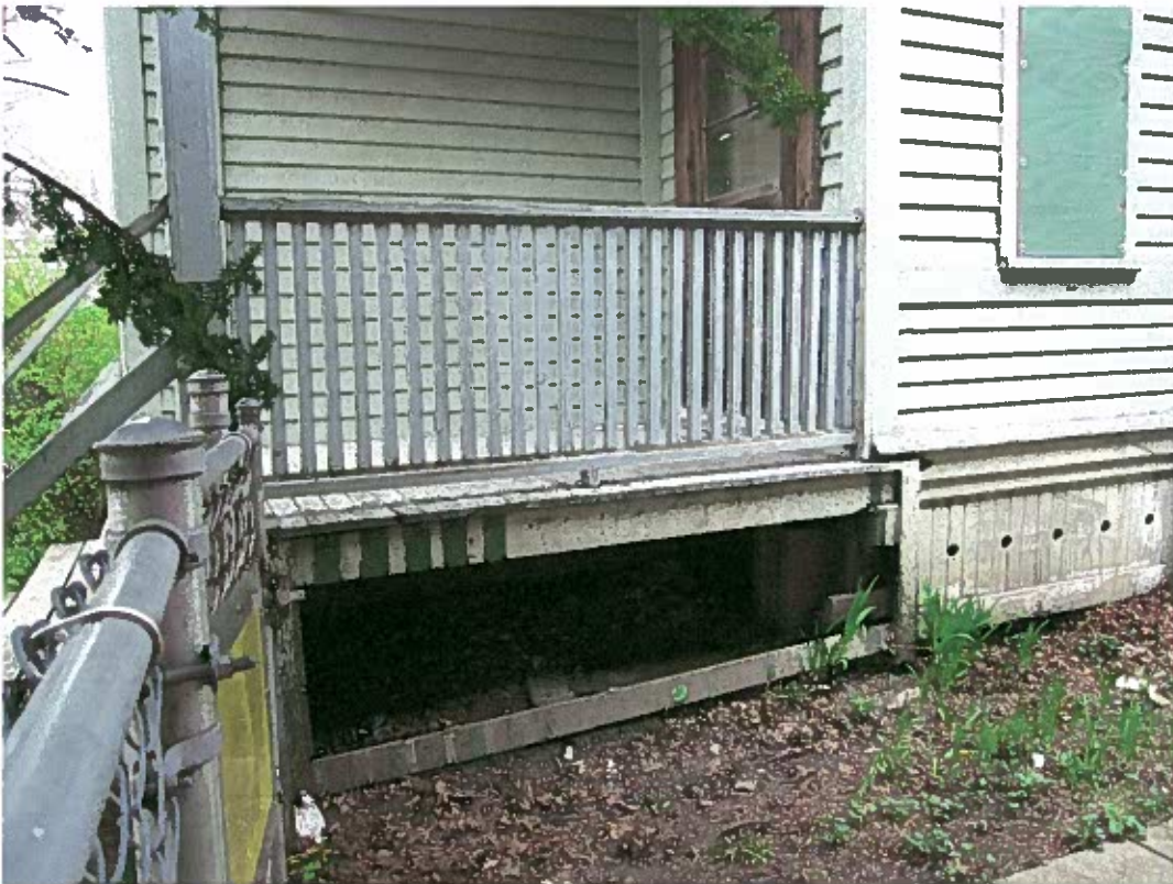
4. Front porch (East Elevation) with missing skirt
