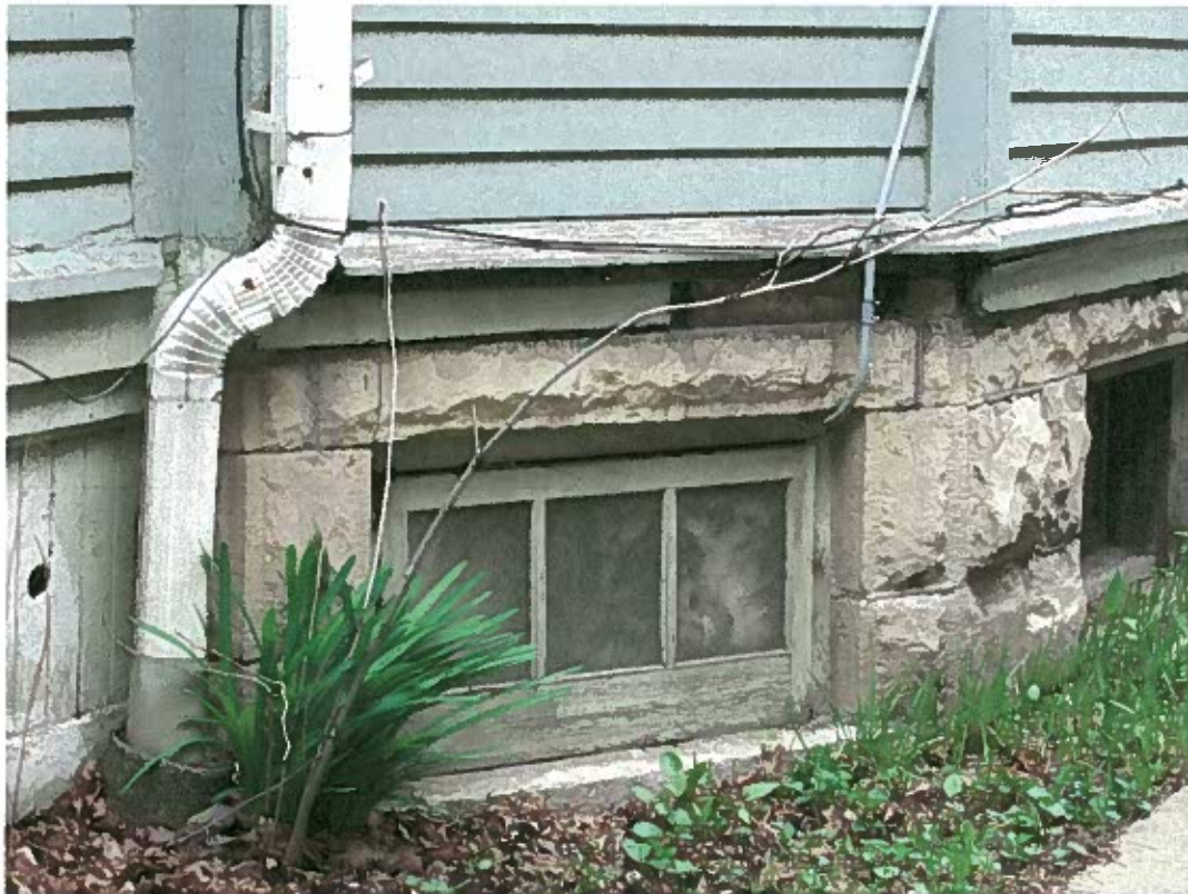
6. Missing Water Table board and drip edge at foundation sill plate
