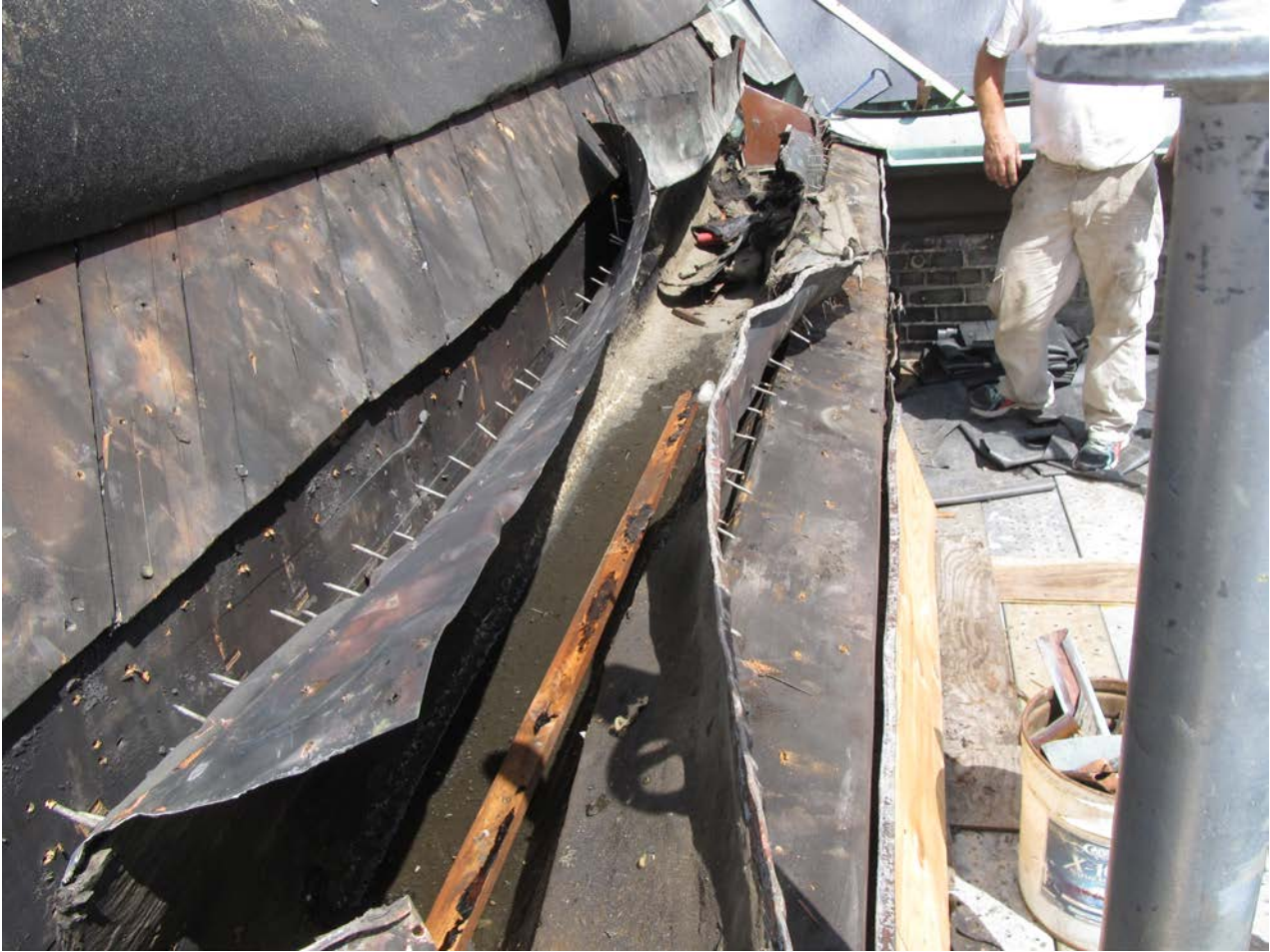
Photo 2 shows removal of the 1972 gutter liner and the later membrane liner, and then exposing the original wood gutter liner bed and top of the original cornice which were left in place.
