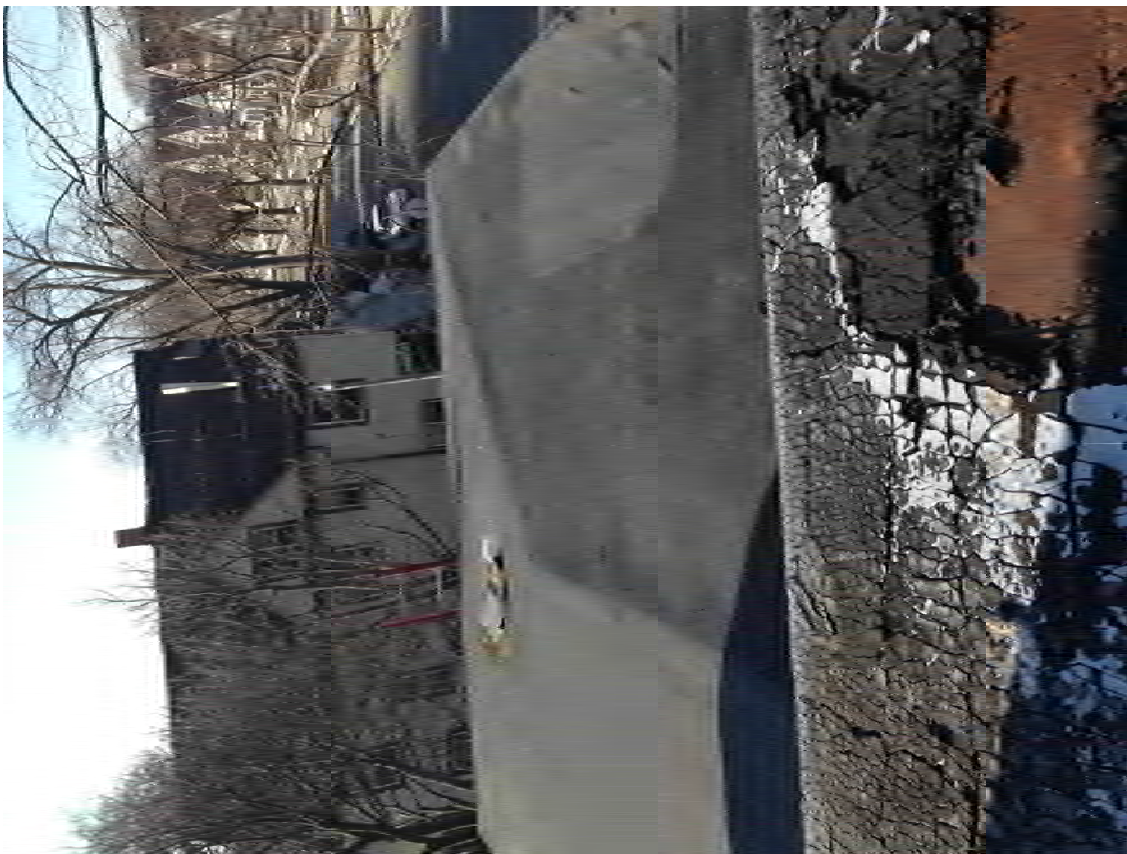
PHOTO 10: Low-pitched hip roof on top of original roof. Deteriorated roof on monitor.
