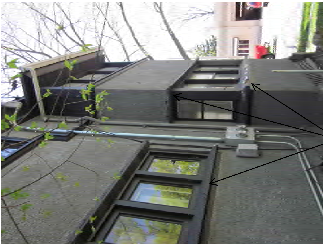
PHOTO 16: Wood trim, in various stages of deterioration/ soundness.
