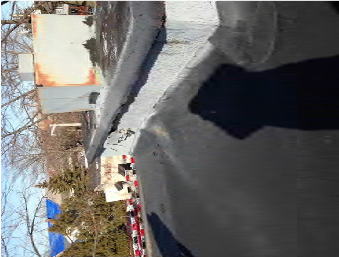
PHOTO 11: Low-pitched hip roof on top of original roof. Deteriorated roof on monitor.
