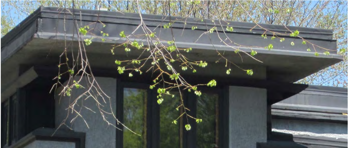
PHOTO 13: Existing fascia condition.
