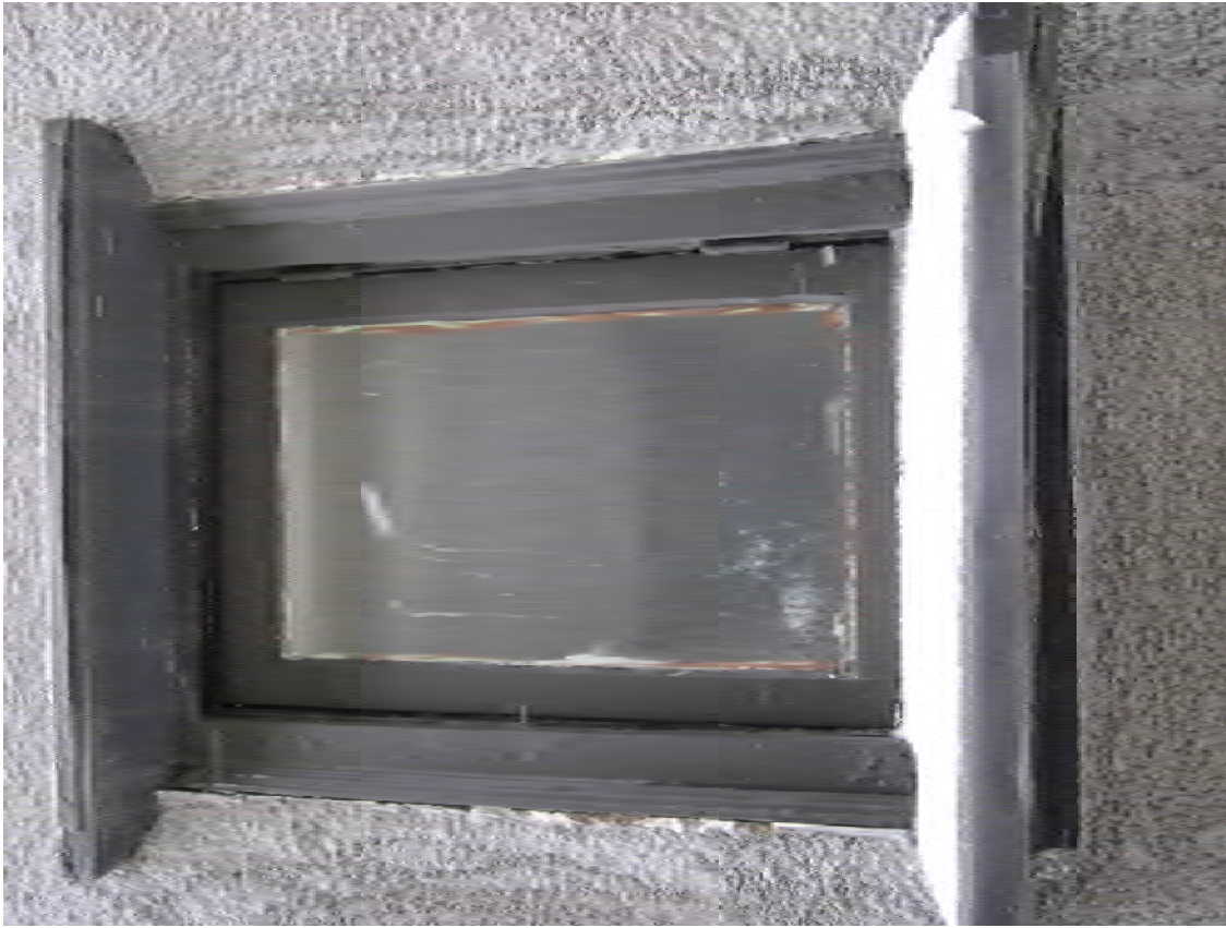
PHOTO 15: Deteriorated wood trim, covered with aluminum cladding.
