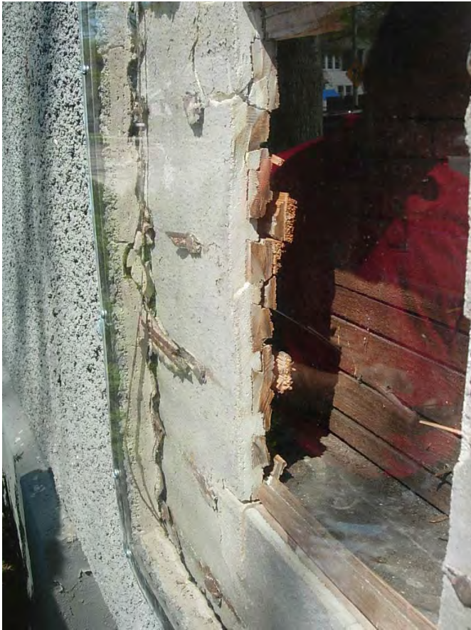
PHOTO 7: Exploratory window in exterior wall showing original and added stucco systems.
