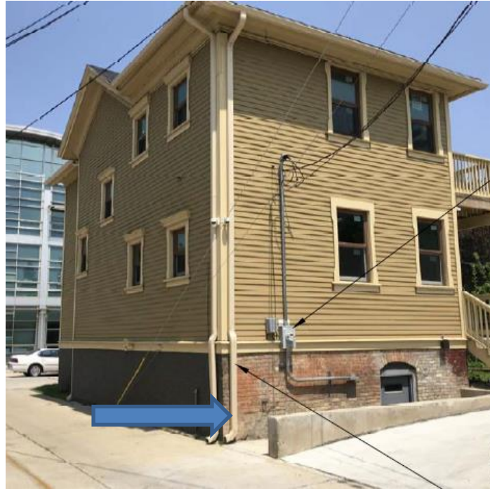
Location on entry enclosure
