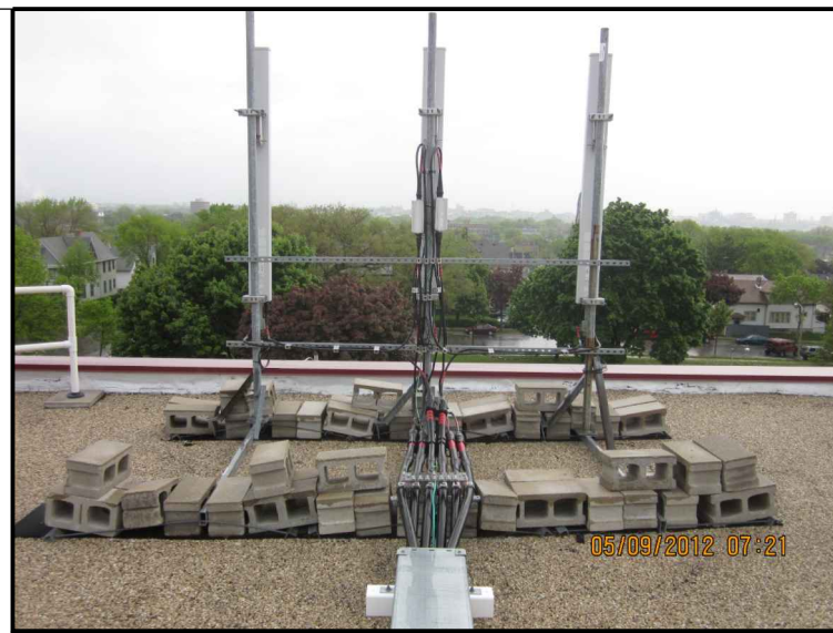
EXISTING T-MOBILE ANTENNAS - ALPHA SECTOR -
