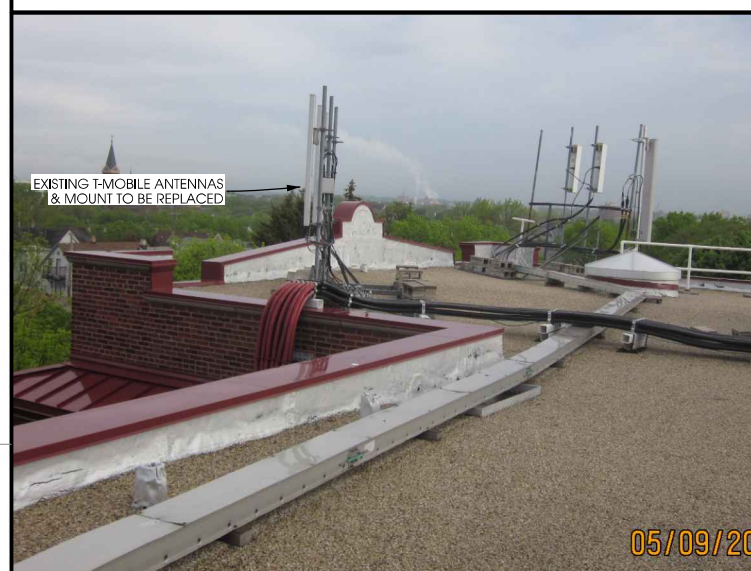
EXISTING T-MOBILE ANTENNAS - GAMMA SECTOR -
