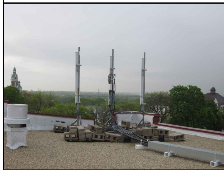
EXISTING T-MOBILE ANTENNAS - BETA SECTOR -
