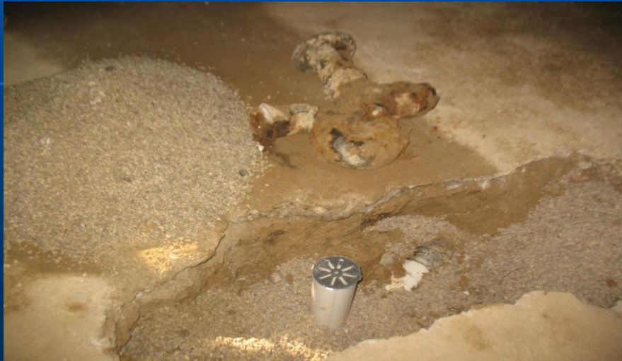
The Palmer Valve in the basement will be removed.
