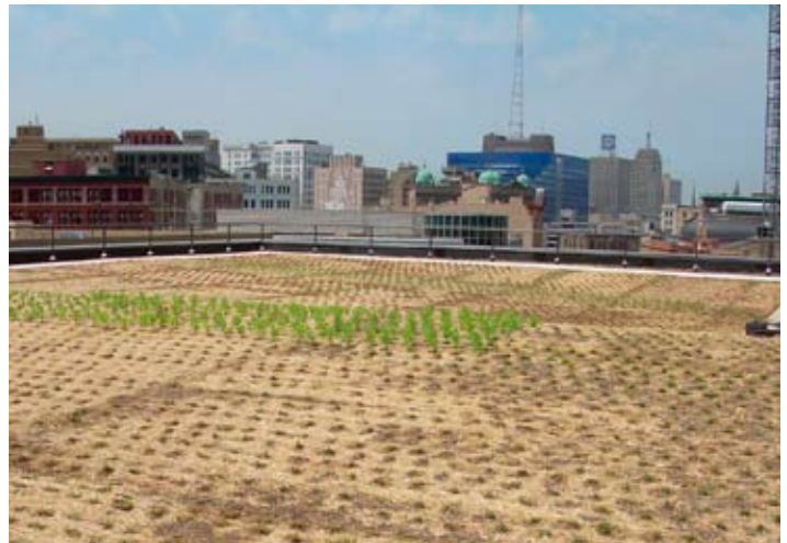
Figure 3.21 Department of City Development - Green Roof
