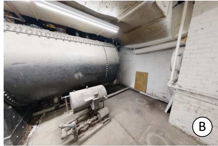
Coal-Fed Boiler at bottom of stairs
