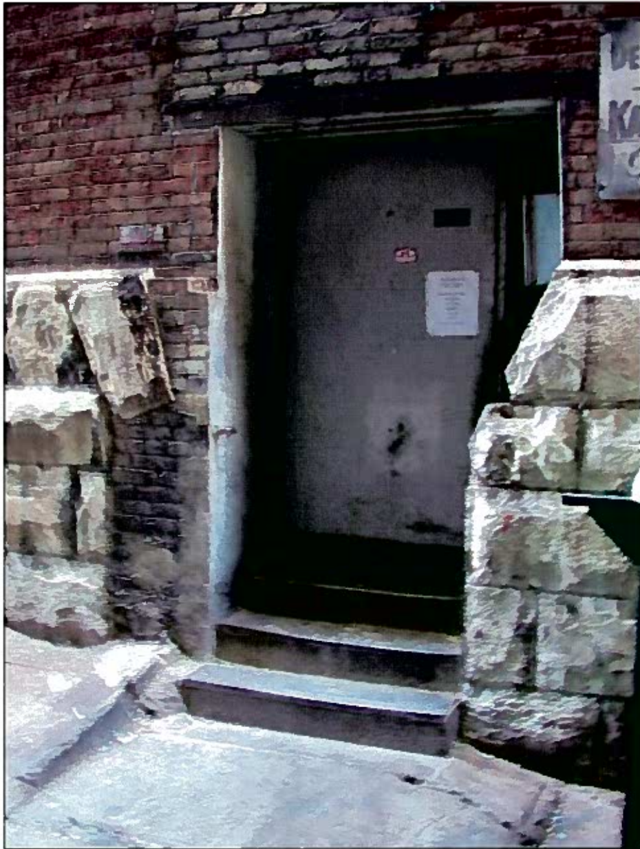
CCF 070632 759 N Milwaukee St 5-5-2008 Looking E across alley at S building entrance in alley
