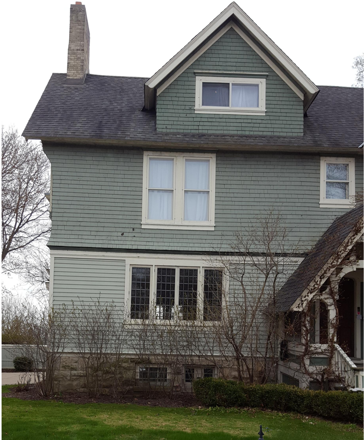
CLOSE-UP OF AFFECTED AREA
