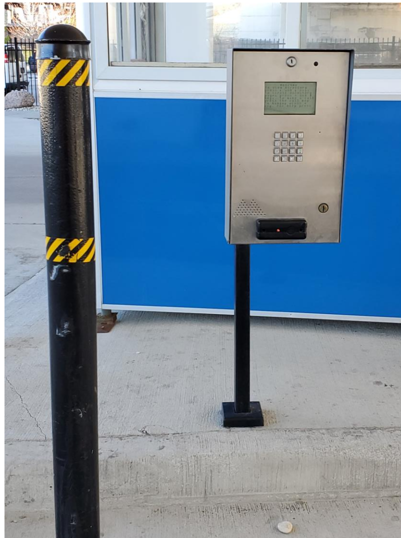
CCF 131802 625 & 640 West Freshwater Way Close up of the security phone.
