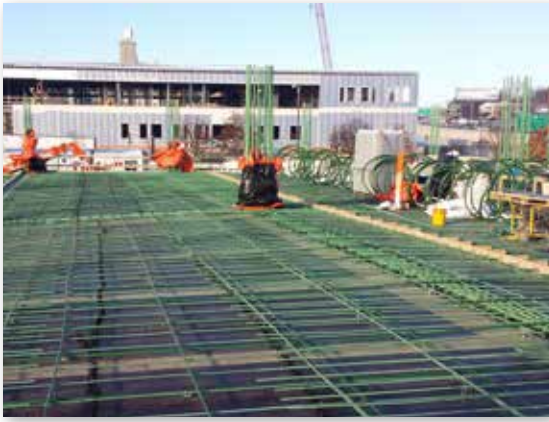
Epoxy coated deck and column rebar installed on the Block 7 Parking Structure by Choice Construction.
