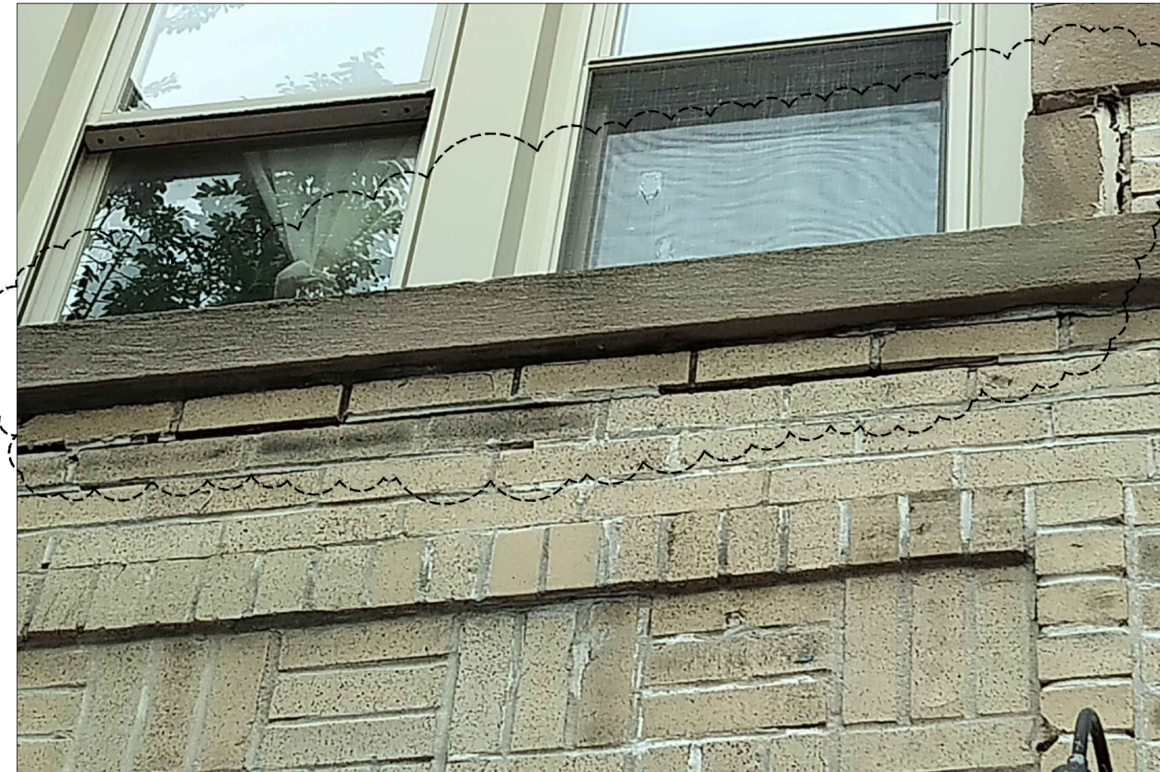
CLOSE UP DETAIL OF THE OPEN JOINTS DO TO MOVEMENT OF WALL
