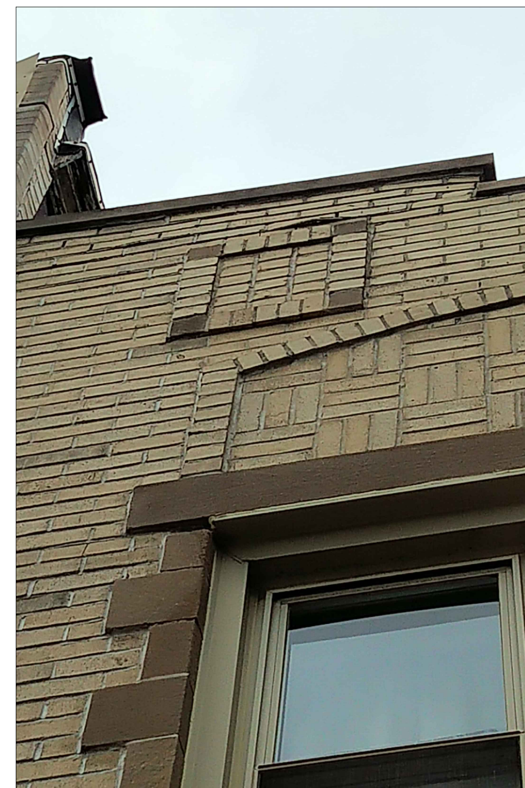
MOVEMENT IS NOTICABLE AT THE PARAPET MORE MORTAR BEING PUSHED OUT OF JOINT
