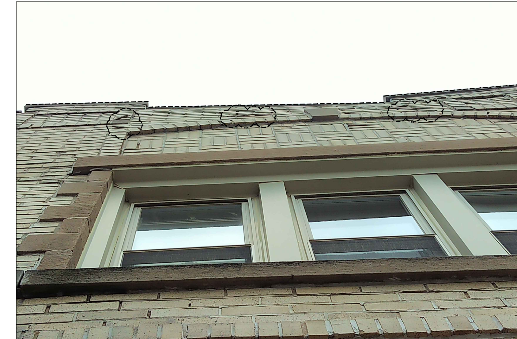
PARAPET ON THE LEFT AND RIGHT ARE AT THE SAME HEIGHT; THERE IS NOTICABLE MOVEMENT AREA OF JOINT MATERIAL BEING PUSHED OUT OF JOINTS.
