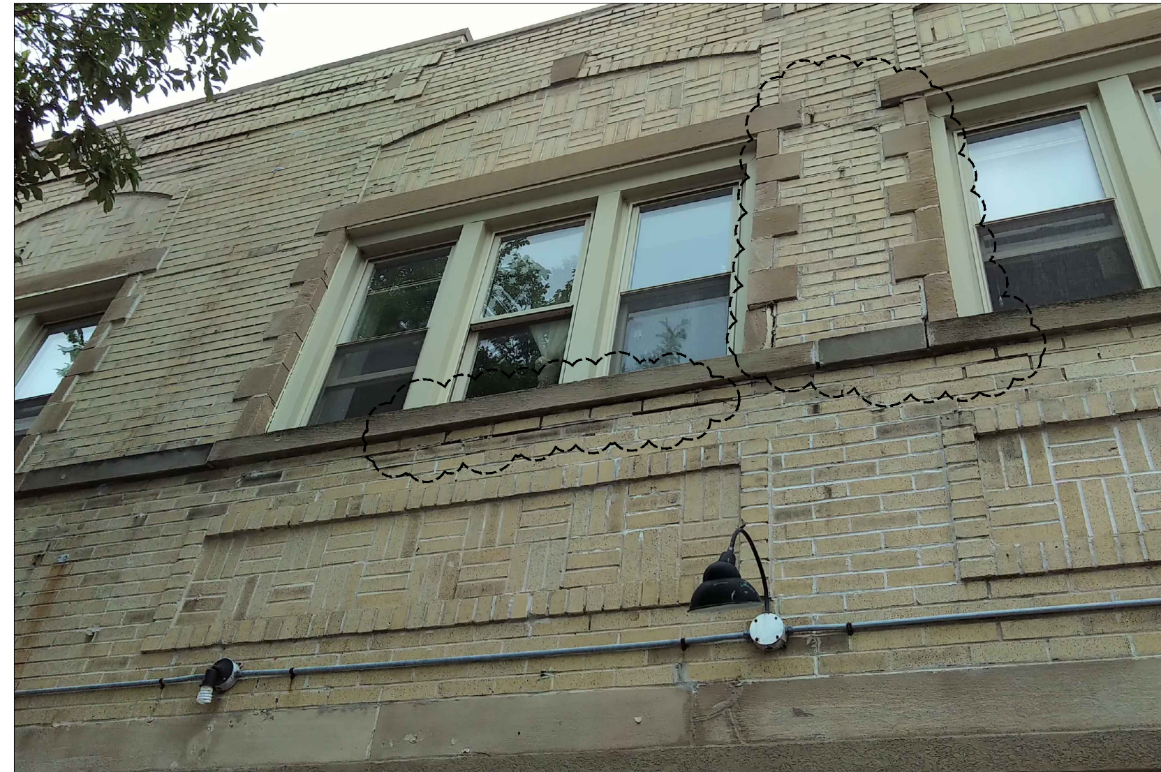
CONSIDERABLE MOVEMENT BETWEEN WINDOWS AND AT THE SILL - MORE OPEN JOINTS
