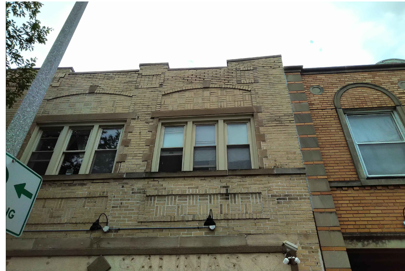
NOTABLE OPEN JOINTS AND MISSING MORTAR; MAJORITY OF BRICK FAILURE IS AT THE LIMESTONE SILL BELOW THE WINDOWS.
