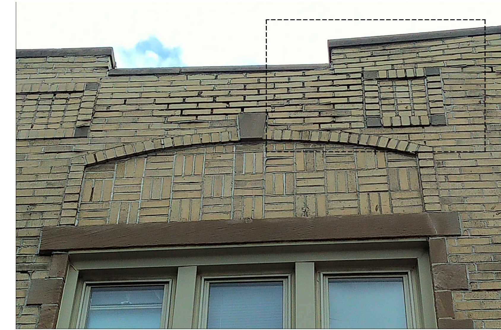
DETAIL ABOVE THE WEST WINDOW - OPEN JOINT AND IMPROPERLY POINTED JOINTS; NOTE THE AREA OF PARAPET MOVEMENT
