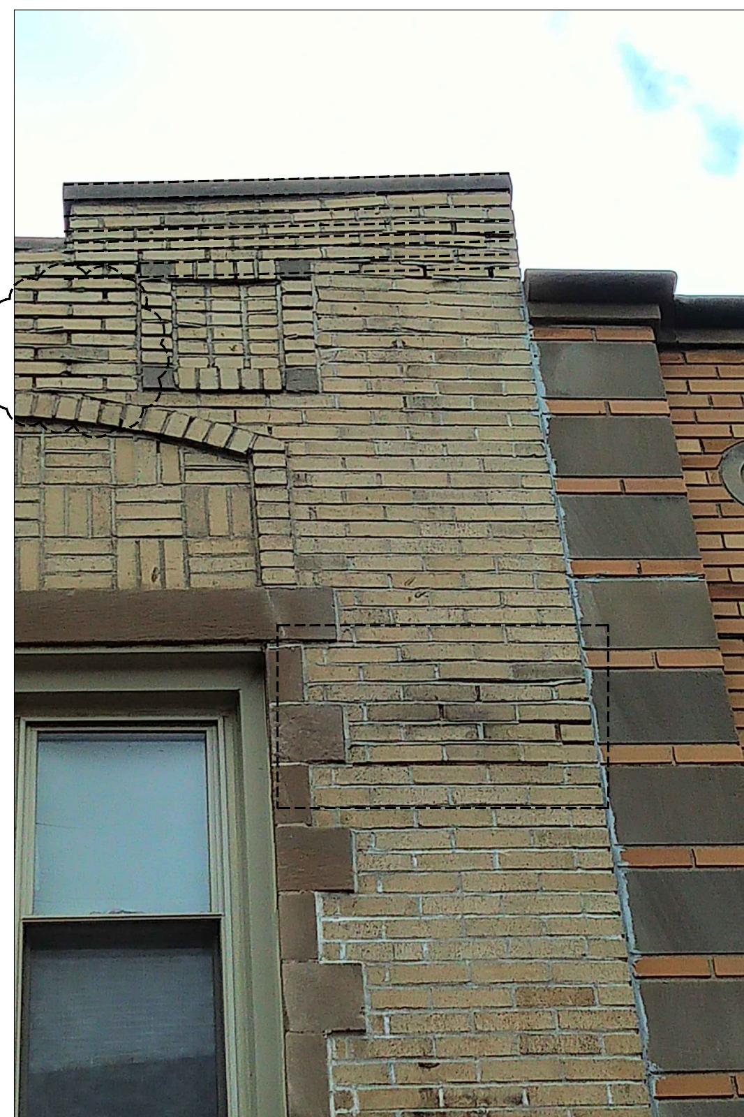
CONSIDERABLE MOVEMENT AT THE PARAPET BRICK MOVEMENT TO THE RIGHT OF THE WINDOW
