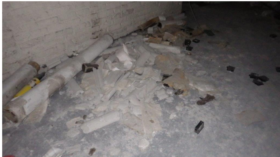
Friable asbestos containing pipe insulation, 2001 West Vliet Street
