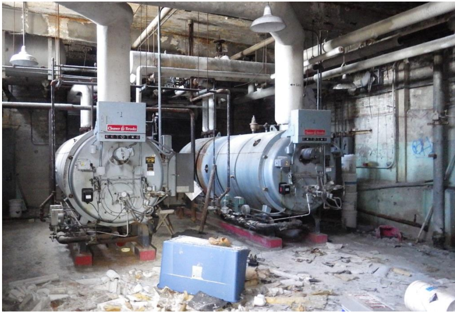
Mechanical Room, 2001 West Vliet Street
