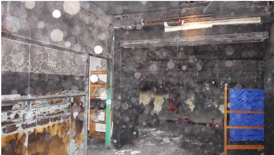
Fire damaged area, airborne particles present 2001 West Vliet Street
