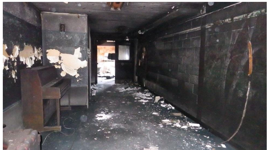
Fire damage, 2001 West Vliet Street
