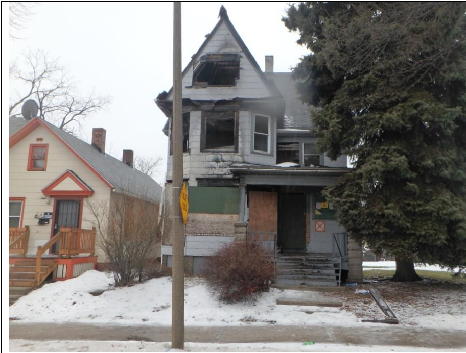
519 North 28 th Street, Fire damaged and demo candidate to be restored with HIPF grant in 2020
