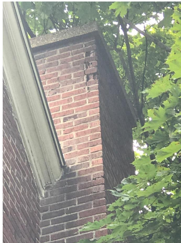
Photos of subject chimney showing damage.
