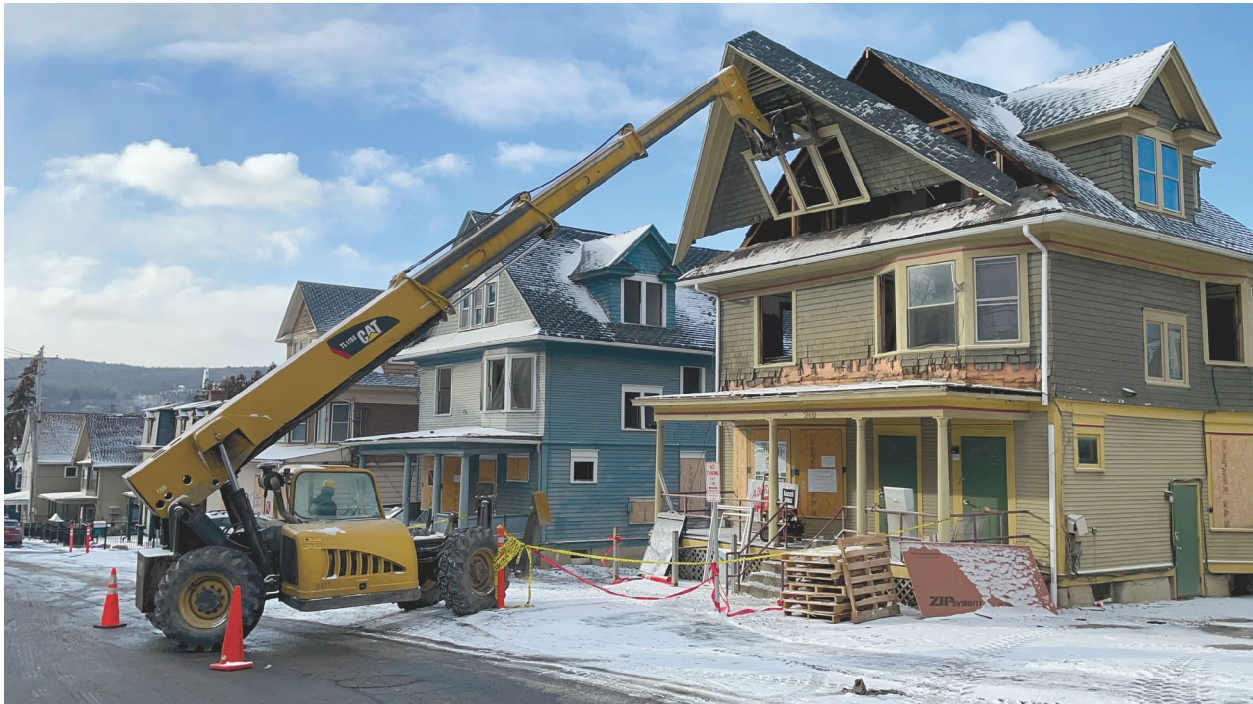
This apartment building in Ithaca, New York, is being deconstructed, piece by piece, as part of a pilot project in sustainable demolition from Cornell's Circular Construction Lab. Photo: Felix Heisel
