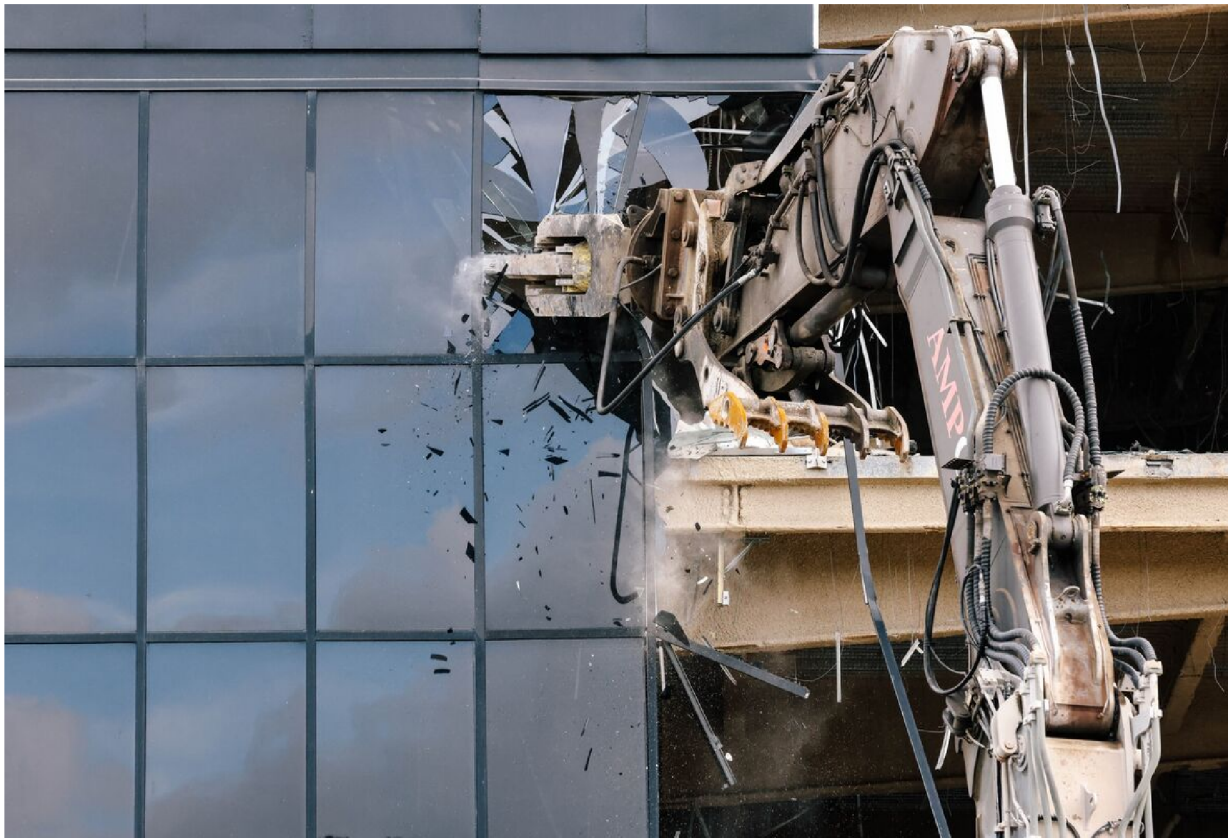
A California office complex built in the 1980s meets an untimely end: demolished to make way for a logistics hub in 2024. Photographer: Dania Maxwell/Los Angeles Times via Getty Images
