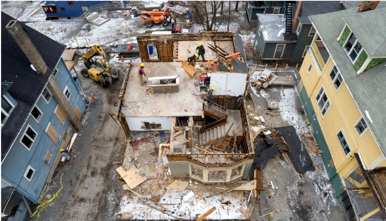
Deconstruction is far more labor intensive than traditional demolition, but the Cornell researchers hope to prove that revenue from reselling materials can compensate for added costs. Photographer: Jason Koski, Cornell University
