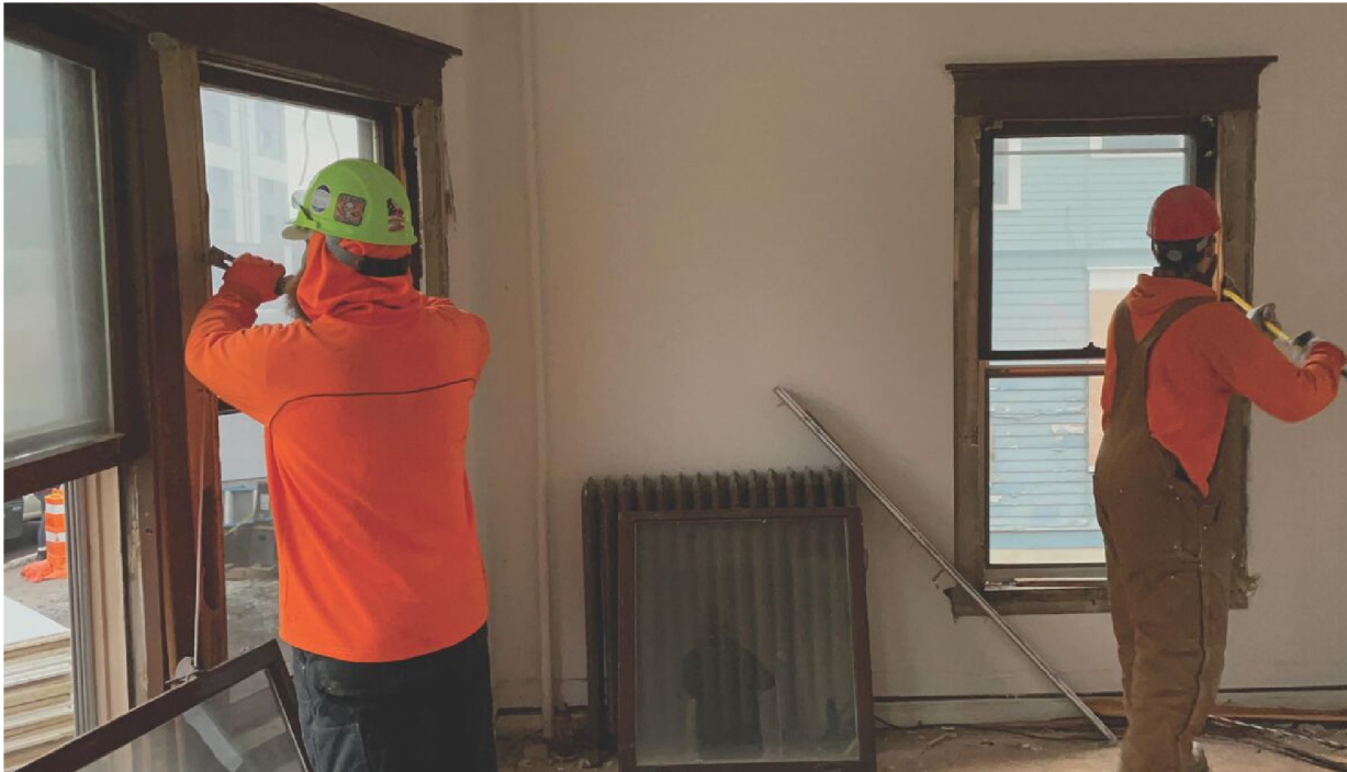
A team of workers removes wooden window frames from 206 College Avenue. Photo: Felix Heisel
