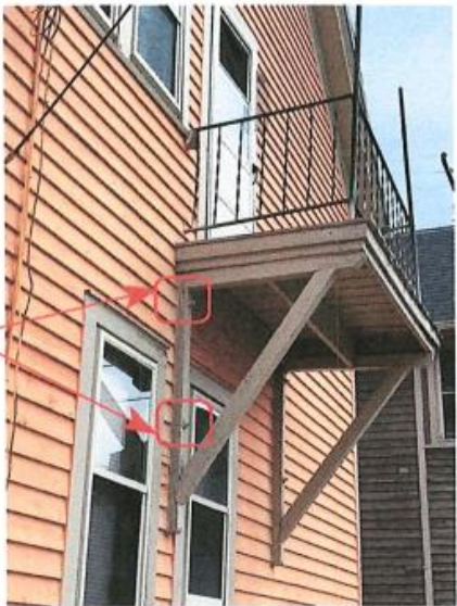
EXISTING PORCH DECK TO BE REPLACED
