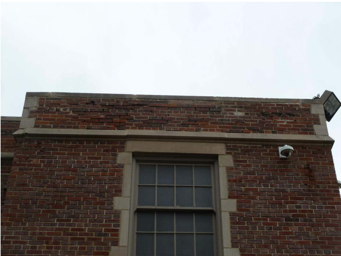
Photo 19 - West parapet damage at Gymnasium
