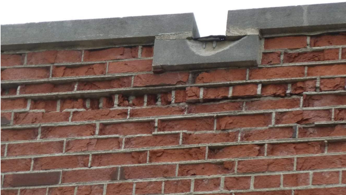
Photo 28 - East parapet damage at Pool Addition
