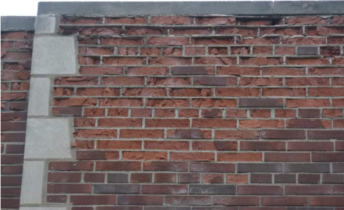
Photo 35 - West parapet damage at Pool Addition
