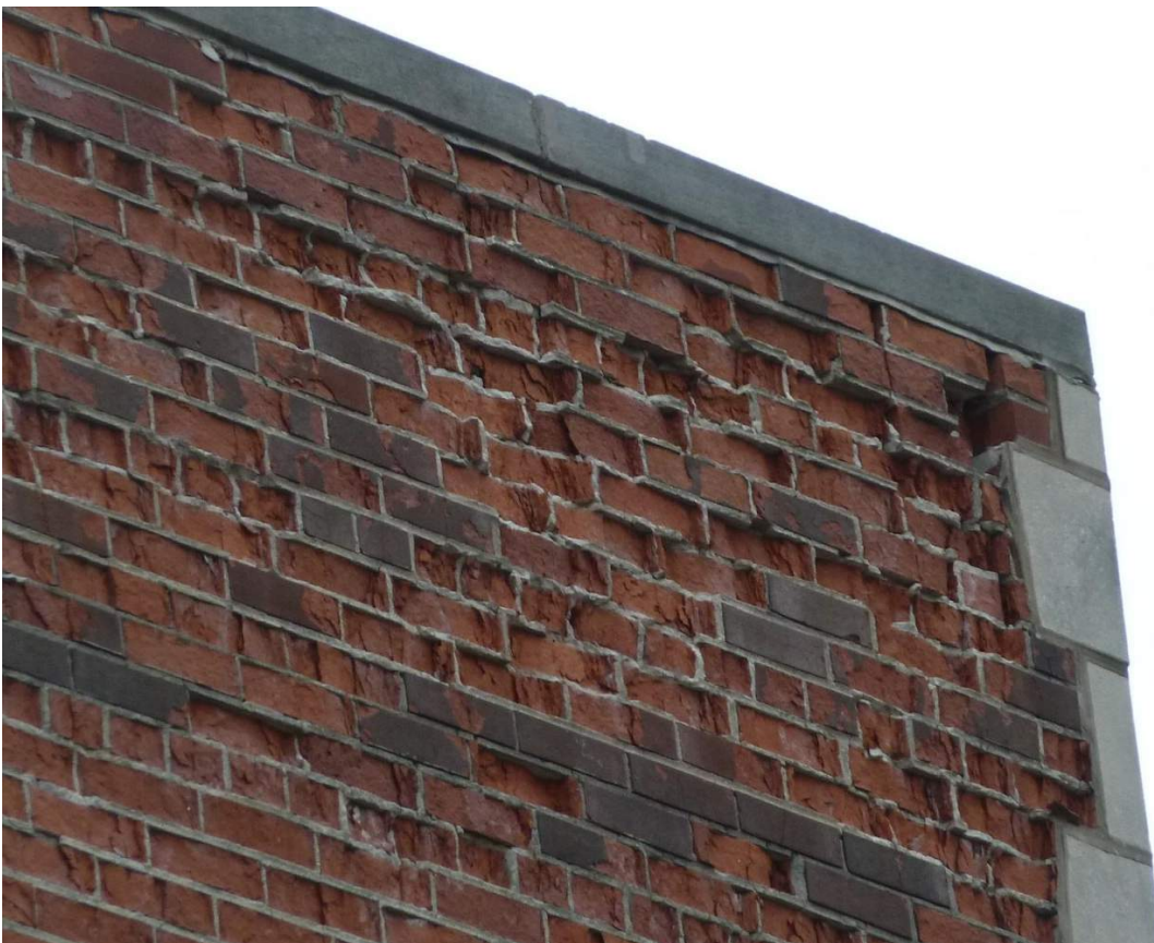
Photo 34 - North parapet damage at Pool Addition
