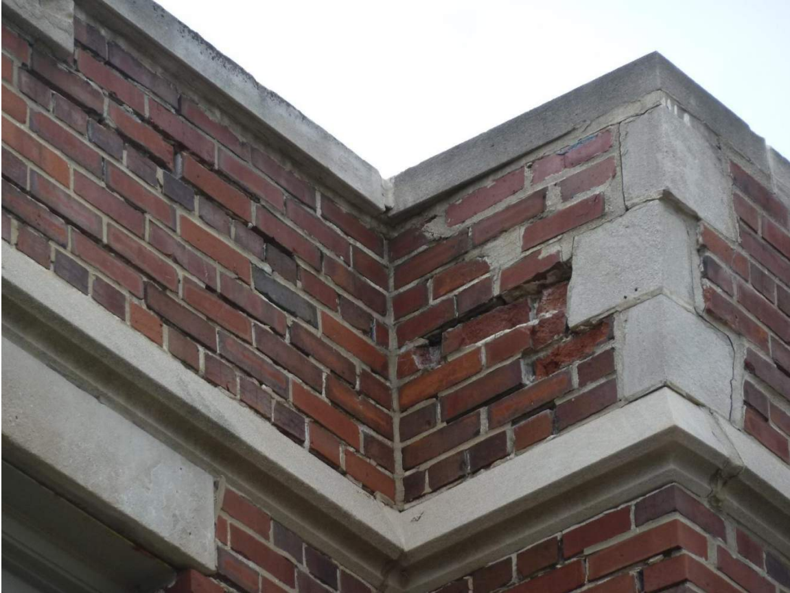
Photo 18 - East parapet damage at Gymnasium
