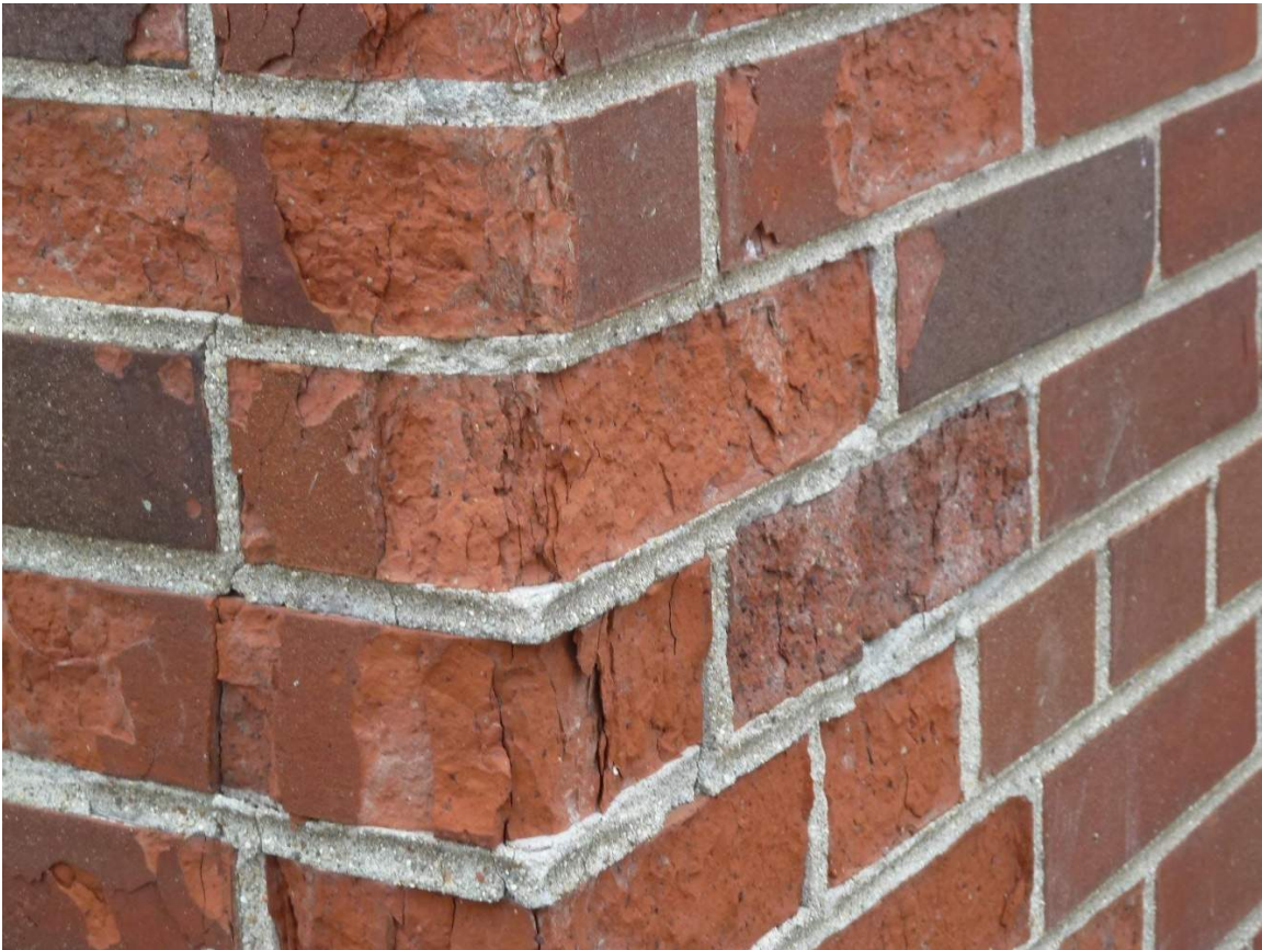
Photo 27 - North-east corner damage at Pool Addition
