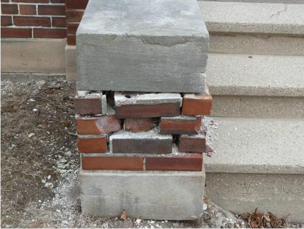
Photo 20 - West entry damage at Gymnasium
