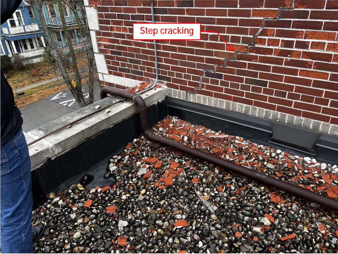
Photo 31 - South-west elevation cracking at Pool Addition
