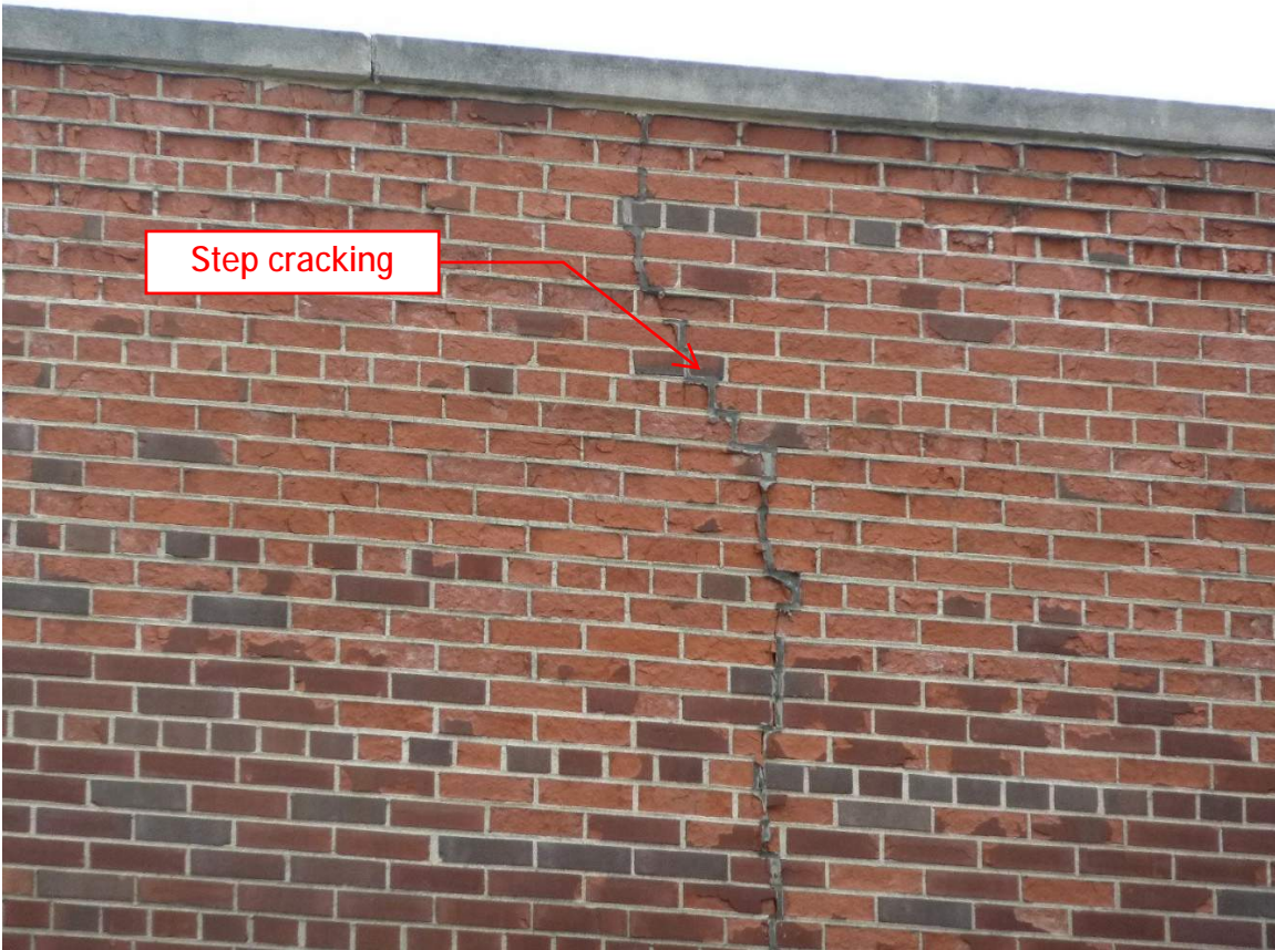
Photo 29 - East elevation cracking at Pool Addition
