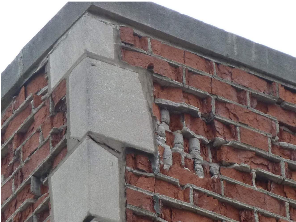
Photo 26 - North-east parapet damage at Pool Addition
