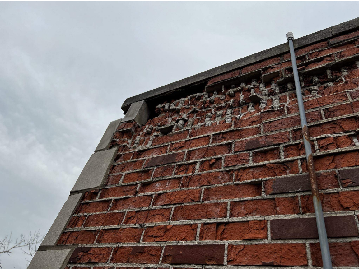
Photo 32 - South-west parapet damage at Pool Addition
