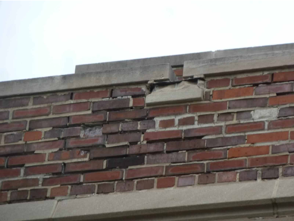
Photo 17 - South parapet damage at Gymnasium
