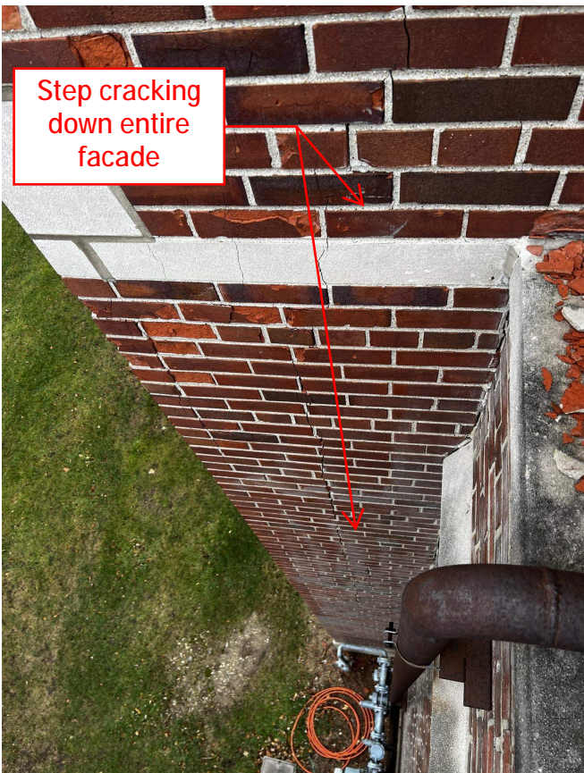
Photo 30 - South-west elevation cracking at Pool Addition
