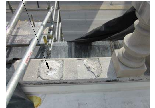
CORRODED MILD STEEL PINS AT BALUSTRADE BASE AND RAIL.
