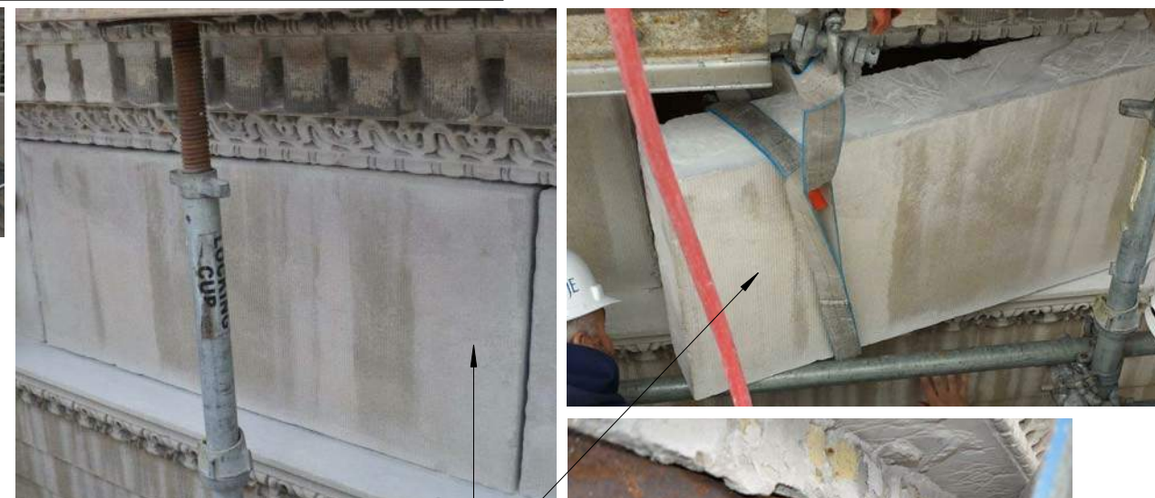
ROTATED FACADE STONE OUTWARD TO VERIFY CONDITION OF STRUCTURAL STEEL CHANNELS, ANCHOR ROD.
