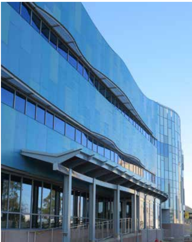
Currently under construction, the UW-Milwaukee School of Freshwater Sciences is a key component of the developing water technology cluster in the city’s Walker’s Point neighborhood. (Source: Department of City Development / Planning)
