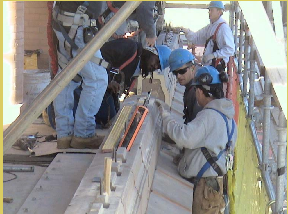
Installation of terra cotta balustrade panel bases on the 12 th floor of the south tower.
