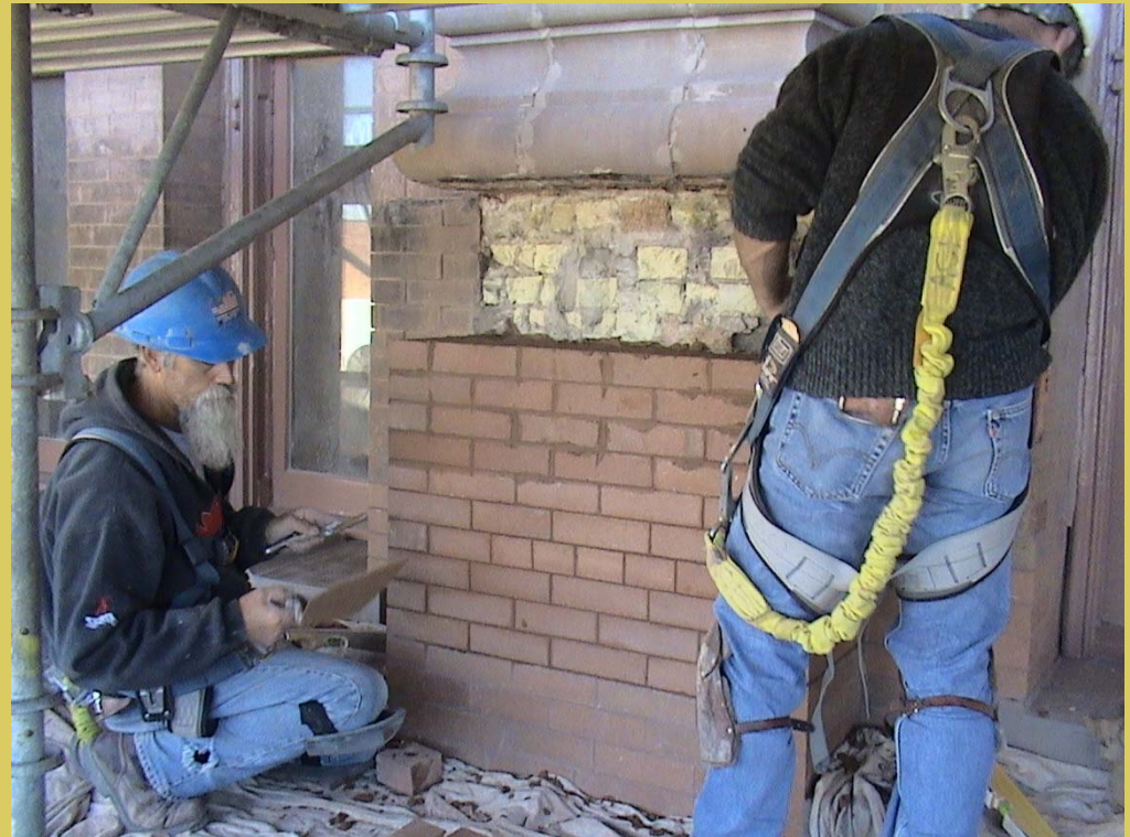
Installation of new face brick between the small dormers on the 8 th floor.
