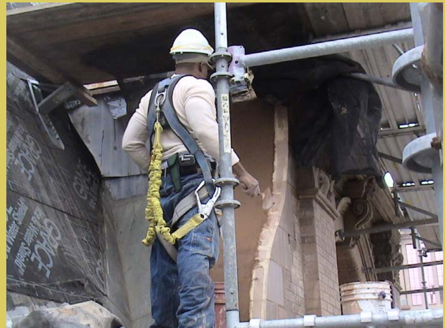
Preparing the existing and new back-up brick for the new terra cotta cap pieces.
