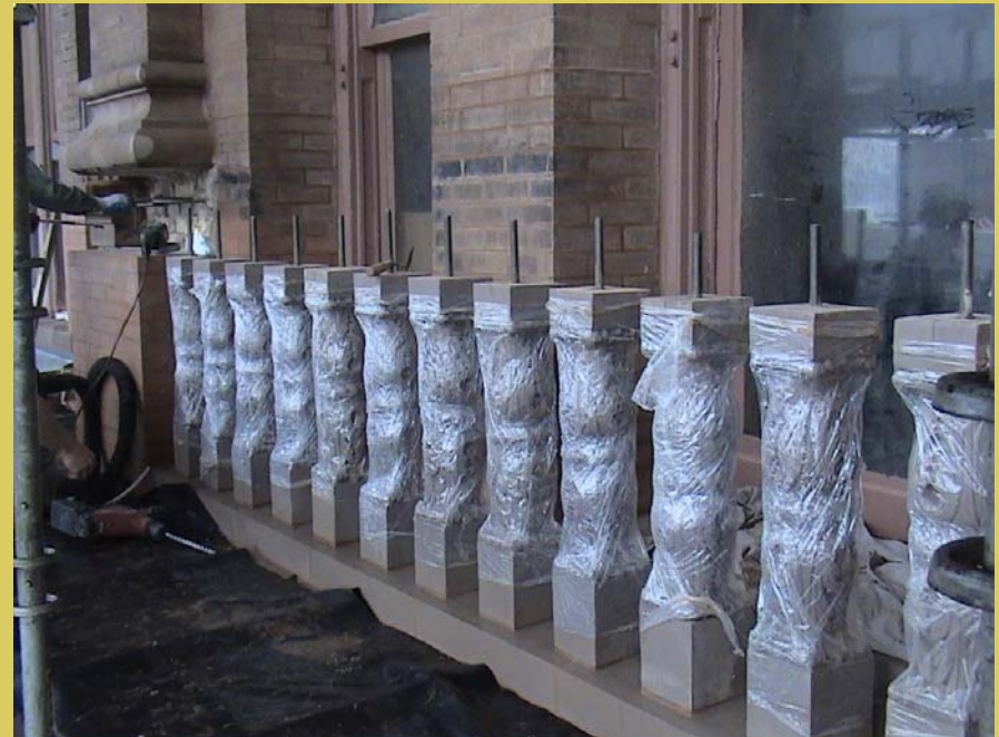
Installation of new balustrade posts on the 8 th floor, center east cross gable.
