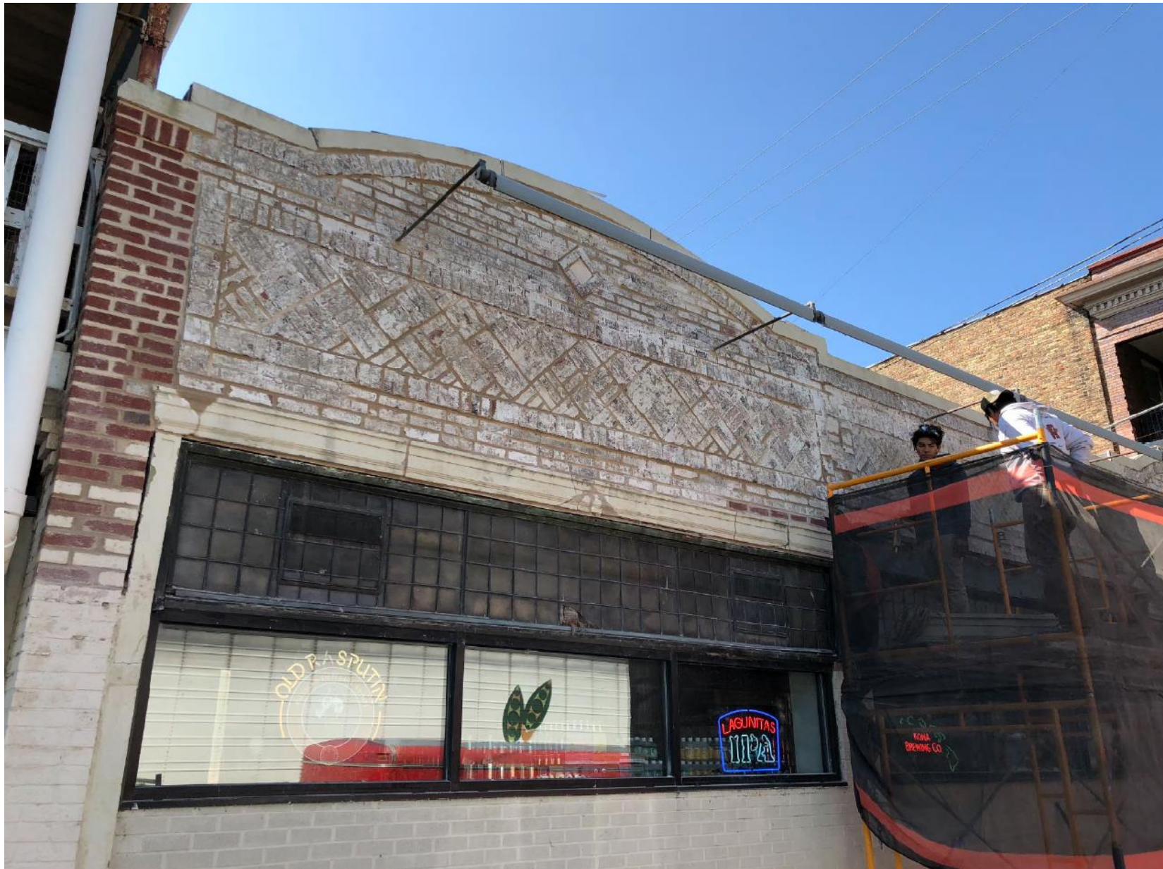
Work in progress showing decorative brick bonding, prismatic glass transom, and structural repairs at lintel and left column
