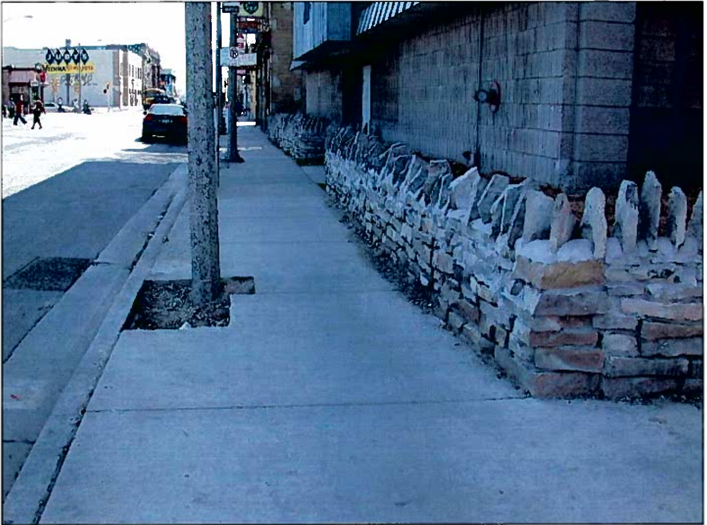
2731 W. Richardson Pl. 071685 5/13/08 Looking south on the west side of North 27th Street at the retaining wall
