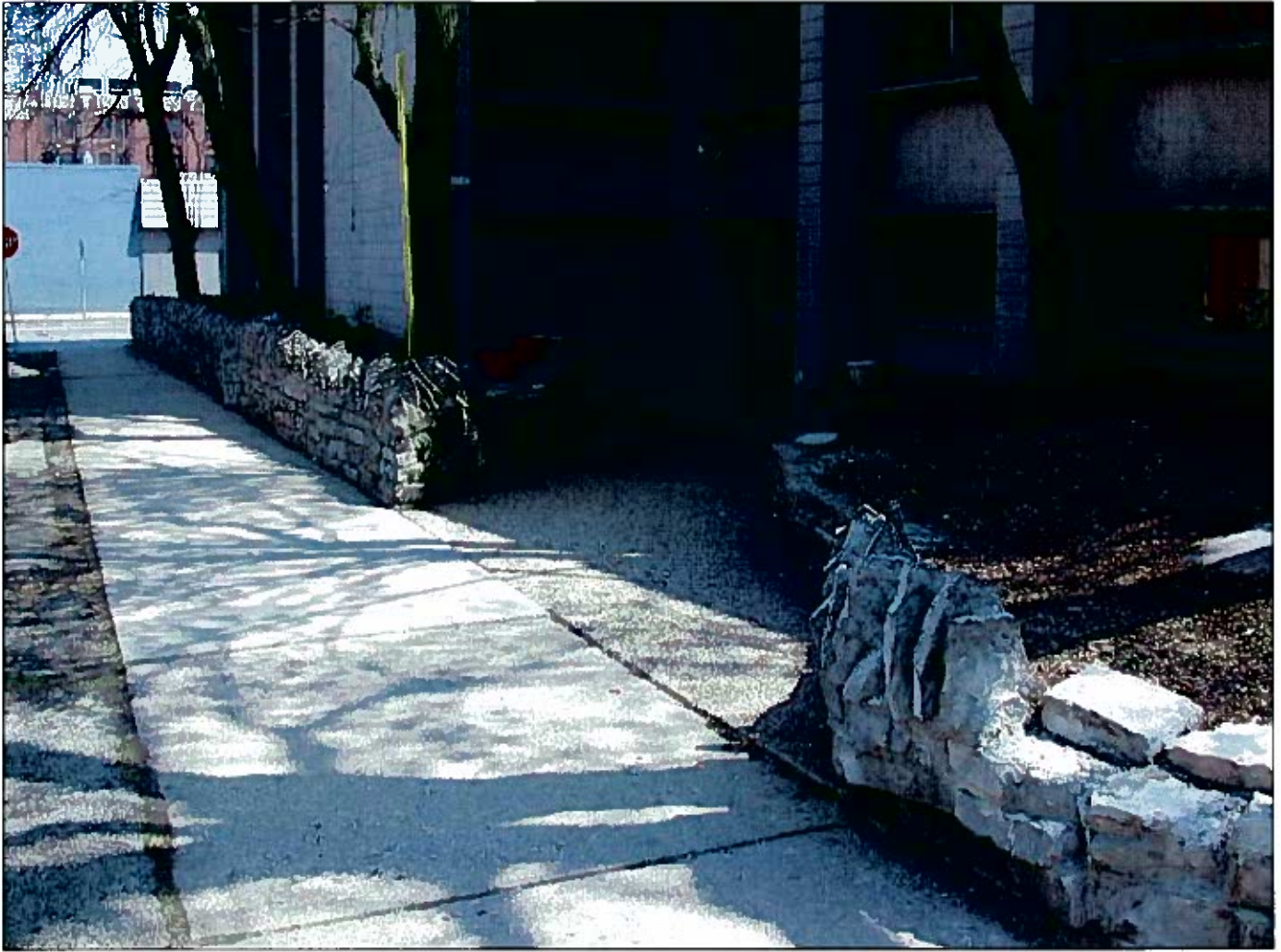
2731 W. Richardson Pl. 071685 5/13/08 Looking east on the south side of West Richardson Place at the retaining wall
