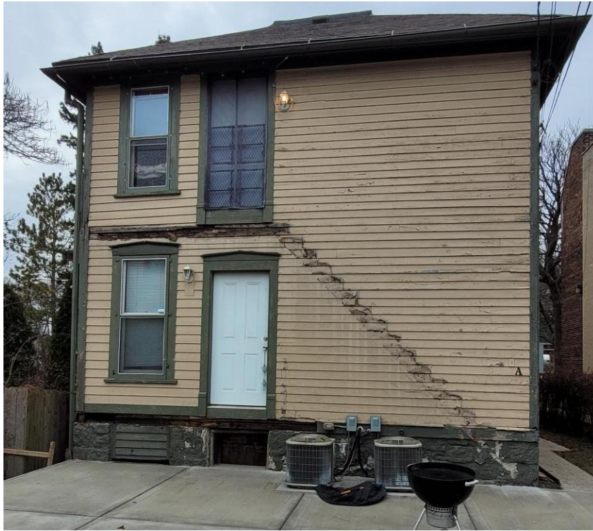
Existing Rear Elevation (After demo) Note existing non-compliant stair rise and run (slope) on paint.
