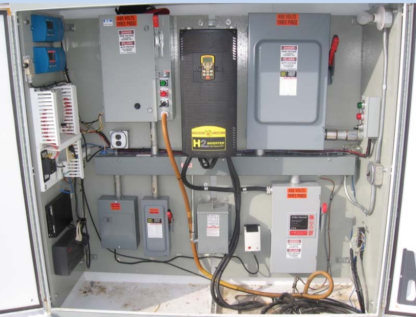
Sanitary Bypass Pump Controls
