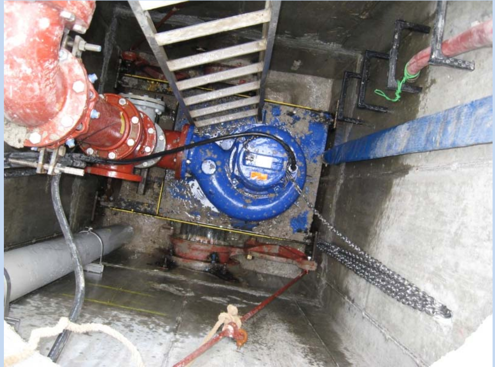
Sanitary Bypass Pump
