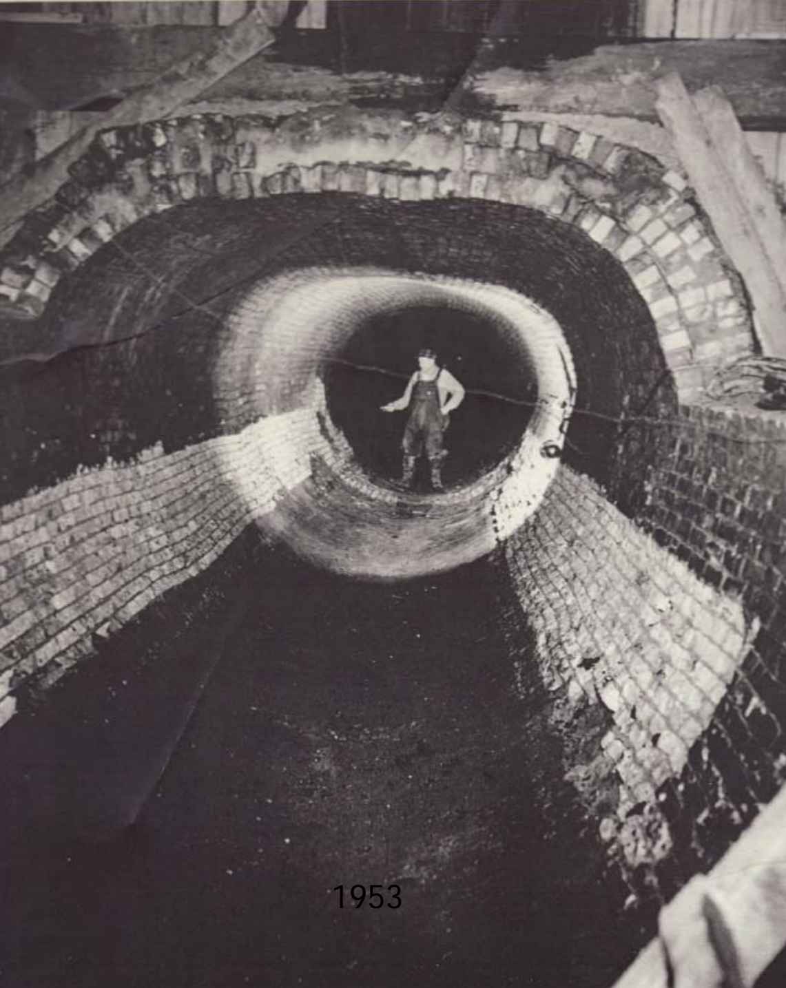
City of Milwaukee West Becher Street 89" and 86" Sewer. Asbestos Bonded Coated and Paved Pipe in a failing brick sewer. The pipe has flattening of its crown and cracks.
