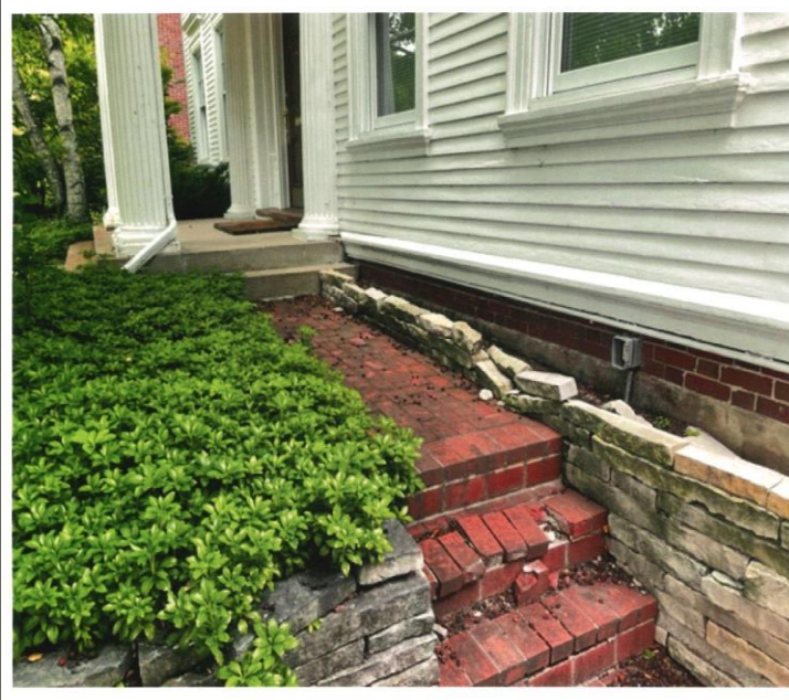
Before crumbling steps and sandstone
