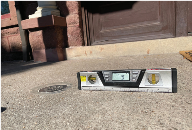
IMAGE 16: Concrete-porch floor slopes away from drain.
