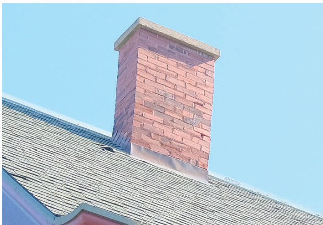
IMAGE 11: Deterioration of the brick and mortar joints on the north chimney is visible from the ground.
