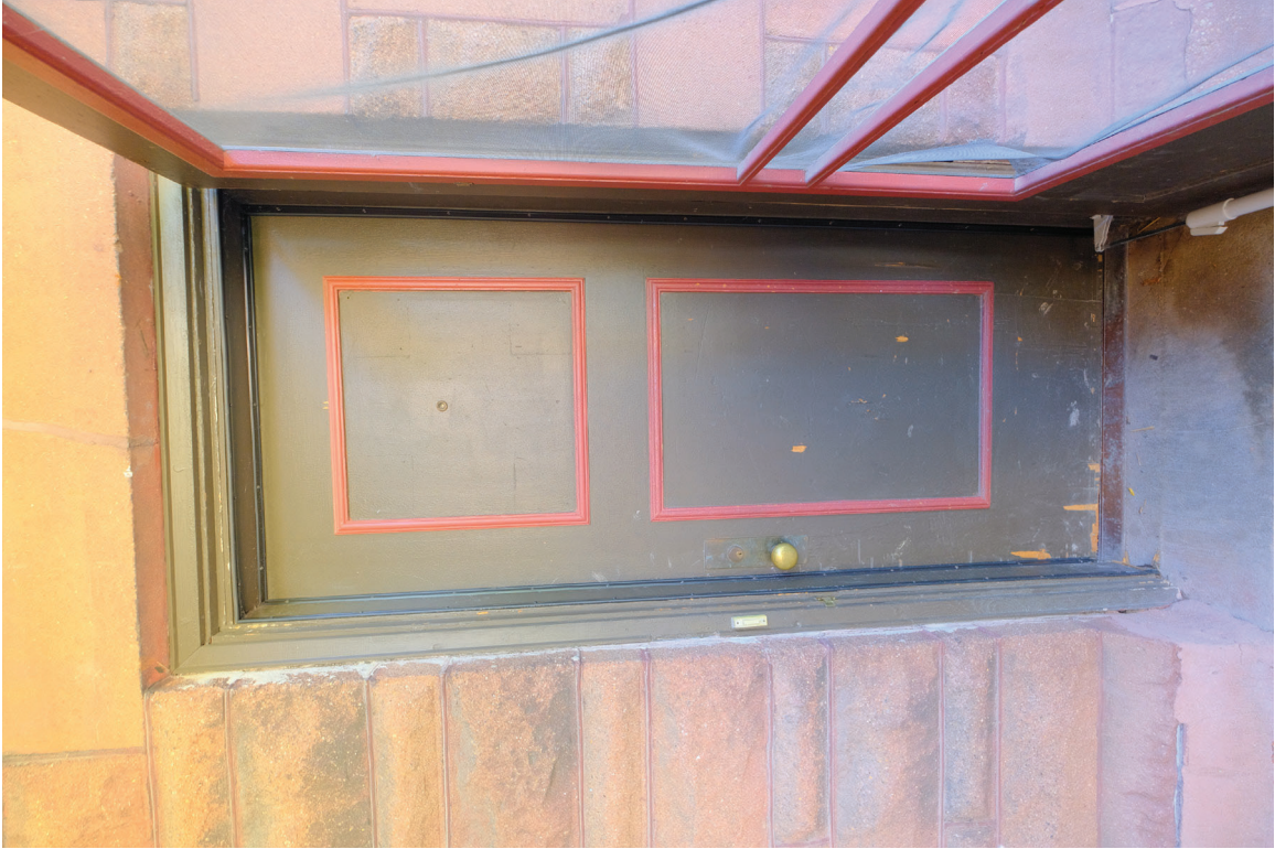
IMAGE 20: West entry door is in poor condition.
