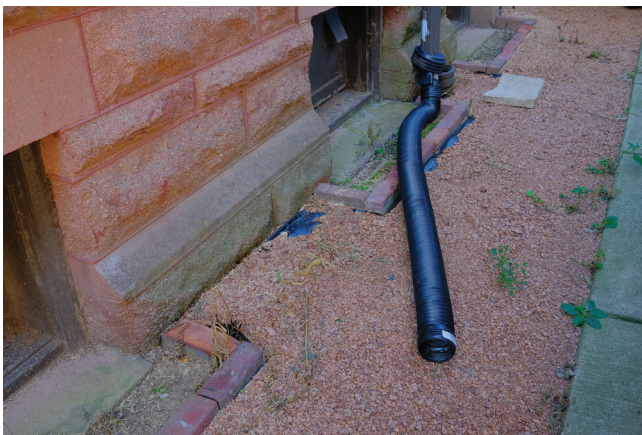
IMAGE 6: Recessed window wells on the north elevation. Downspout-extension outlets too close to the foundation, exacerbating moisture accumulation and algae growth.
