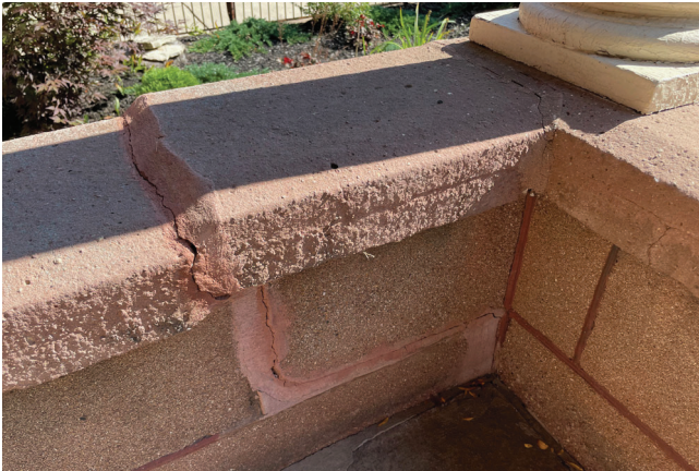
IMAGE 15: Cast-stone units have shifted significantly over time. Note the evidence of previous repairs.
