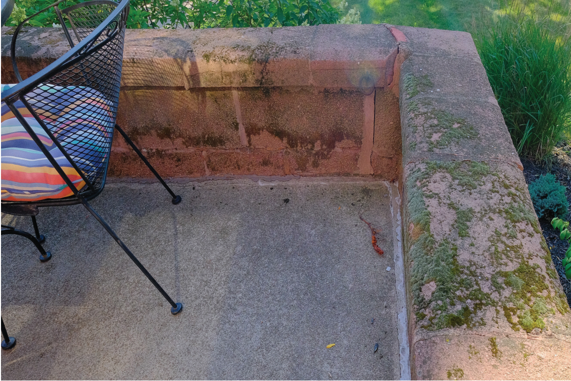
IMAGE 13: Algae has begun to grow on some porch surfaces. Note the evidence of shifting cast stone units and cracking in floor slab. Previous repairs are also evident.
