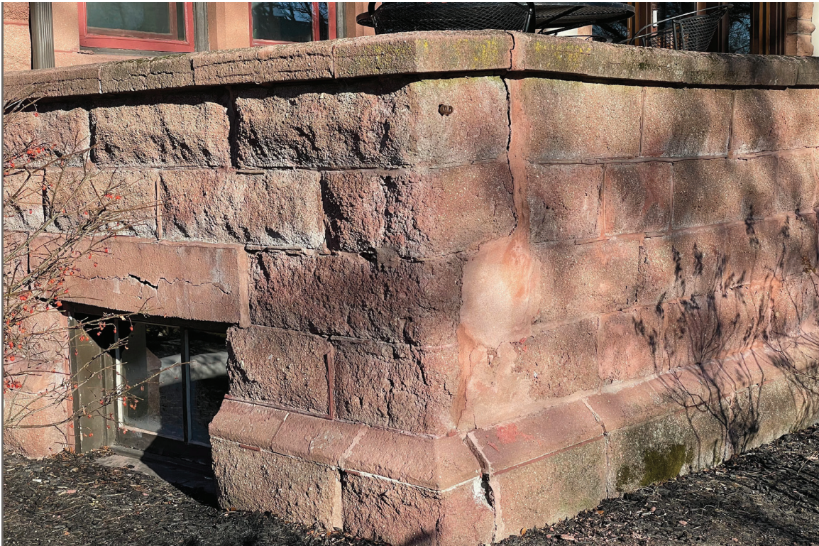
IMAGE 14: Some cast-stone units and open mortar joints have been replaced and attempts at repairs have been made. Shifting and algae growth are visible.
