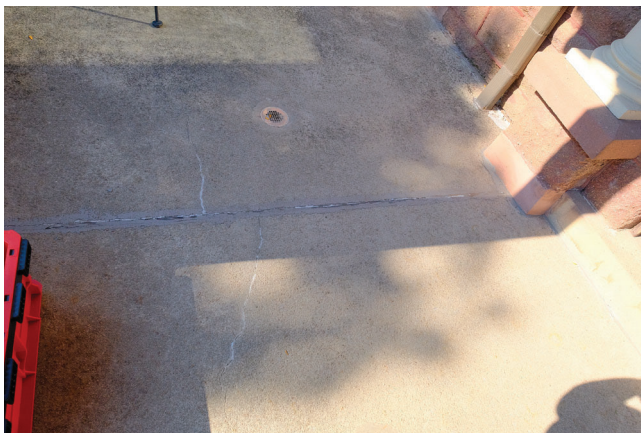
IMAGE 17: Cracking in the concrete-porch slab.
