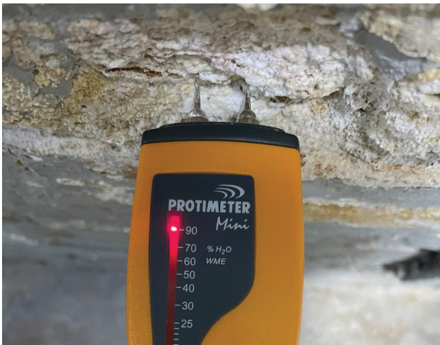
IMAGE 8: High moisture-meter readings along the perimeter walls in the basement.
