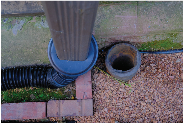
IMAGE 7: Algae growth at the base of the north elevation near downspout.
