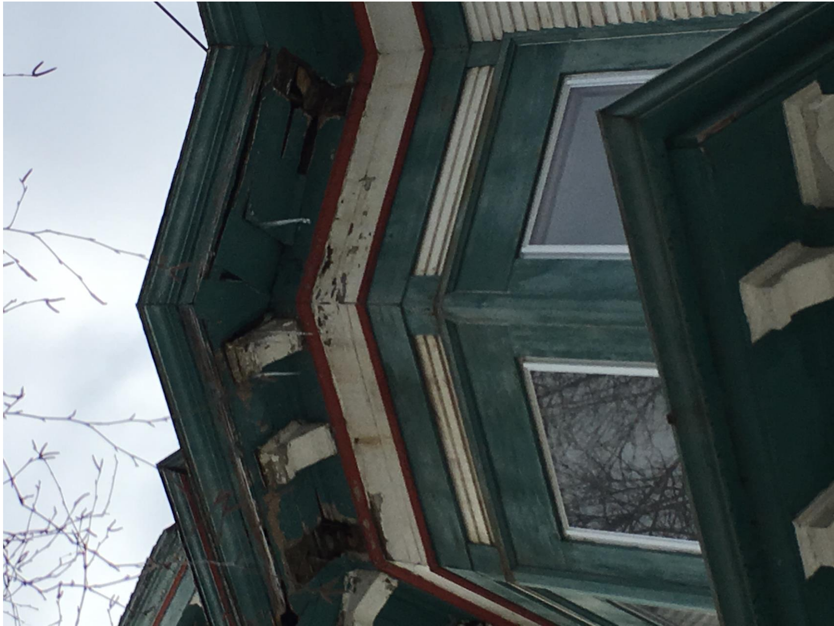
Typical roofline damage
