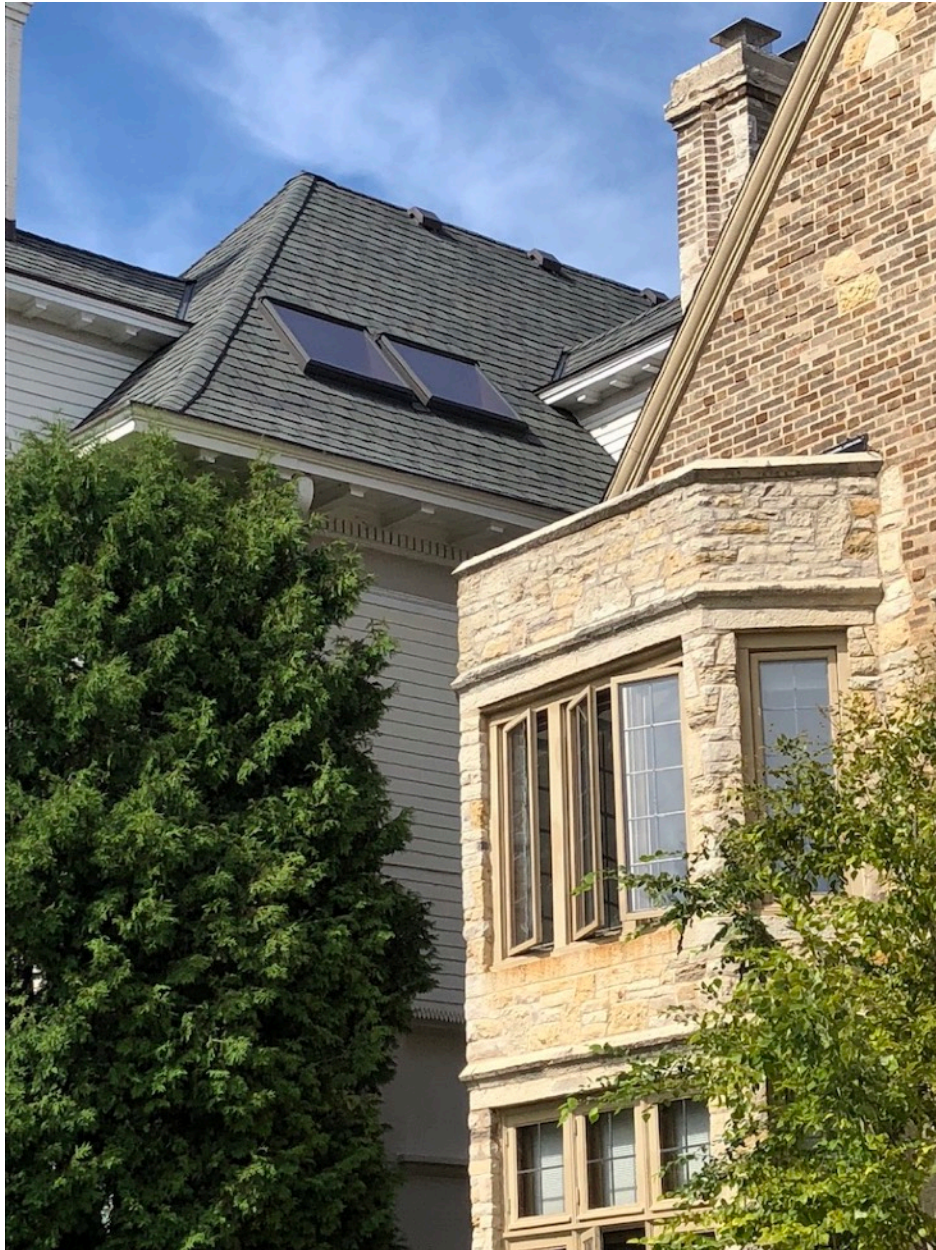
View of side facing skylights at 2064 N Terrace—from same side of street
