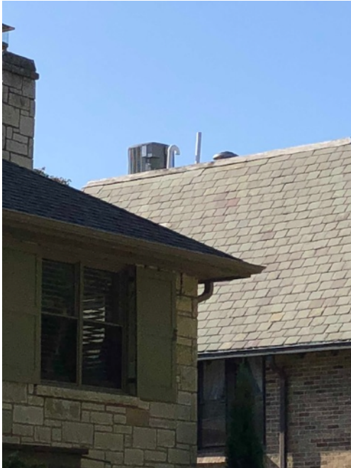
Roof mounted A/C appliance and other pipes & protrusions at 2370 N. Terrace
