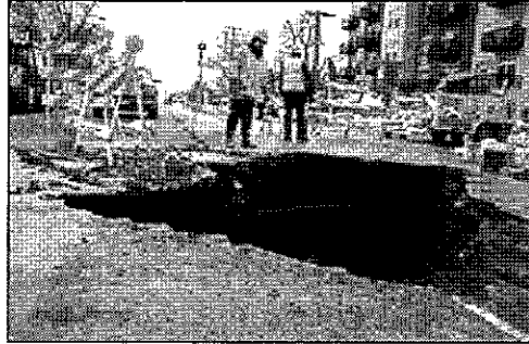
City of Milwaukee sink hole February 2009
