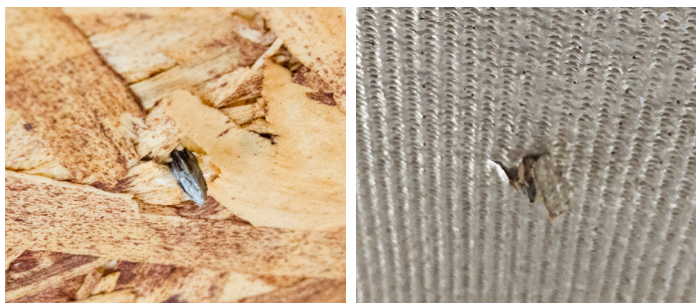
Roofing nails piercing roof decking
