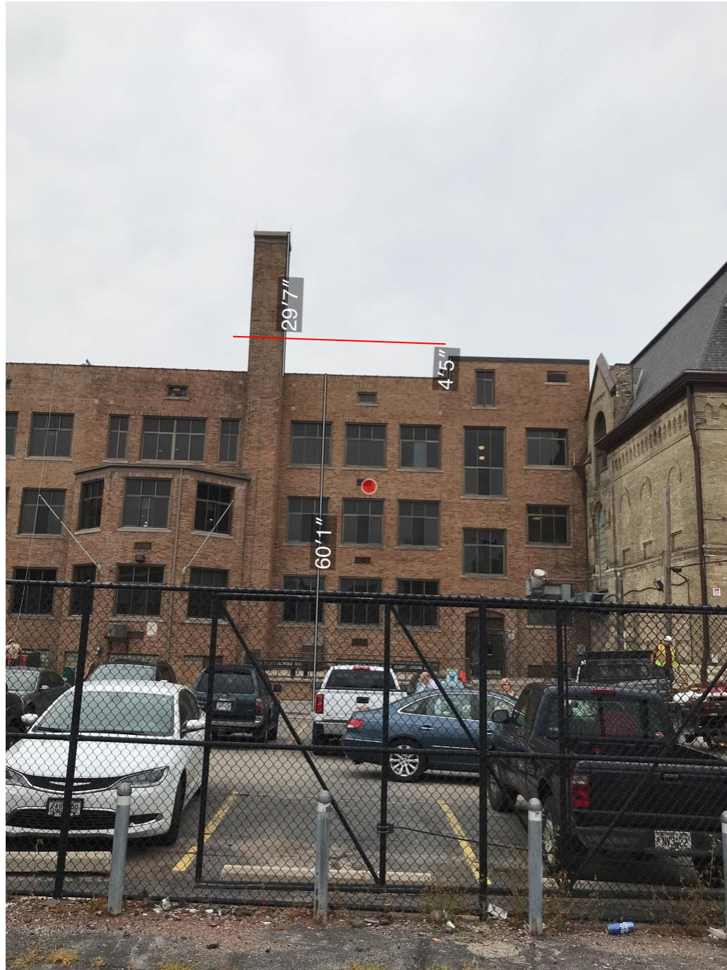
Approximate measurements on rear elevation. Red line shows approximate height of shortened chimney.
