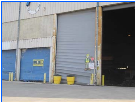
Garage door at west elevation is collapsed
