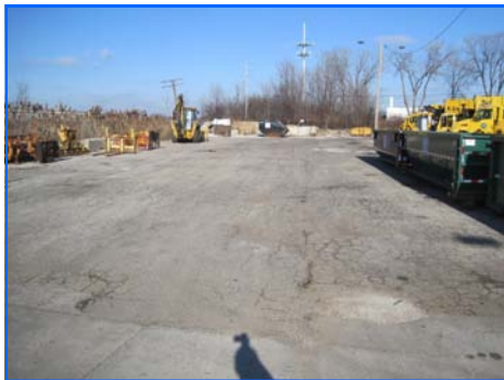
Pavement requires maintenance
