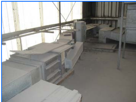
AHU - note accumulation of particulate matter
