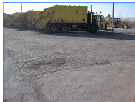
Failed pavement at west end of property
