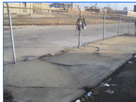
Large unsealed cracks at MRF asphalt pavement
