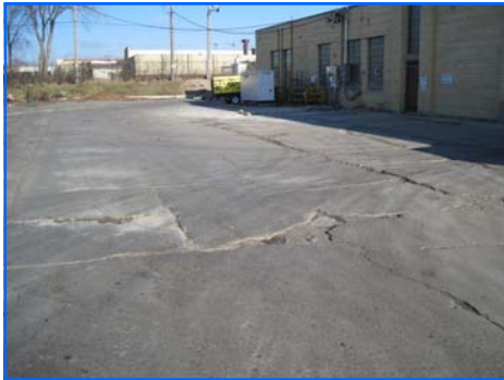
Deteriorated concrete at west end of garage
