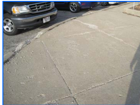
Deteriorated concrete and curbs
