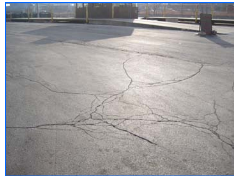
Large unsealed cracks at MRF asphalt pavement
