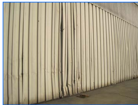
Damaged siding at south elevation
