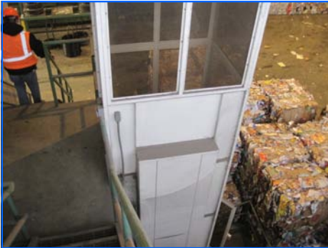
Single passenger elevator
