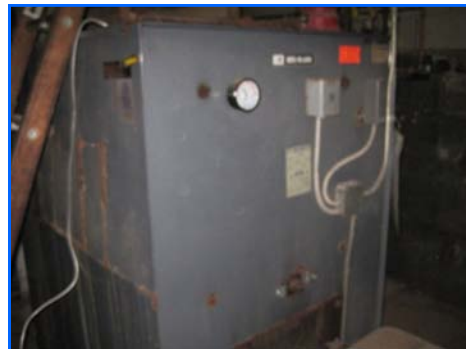
Building heat boiler
