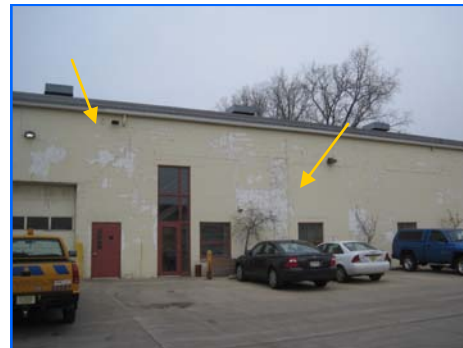
Paint finish deterioration at the Central HQ Building
