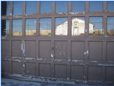
Typical garage door with paint finish deterioration
