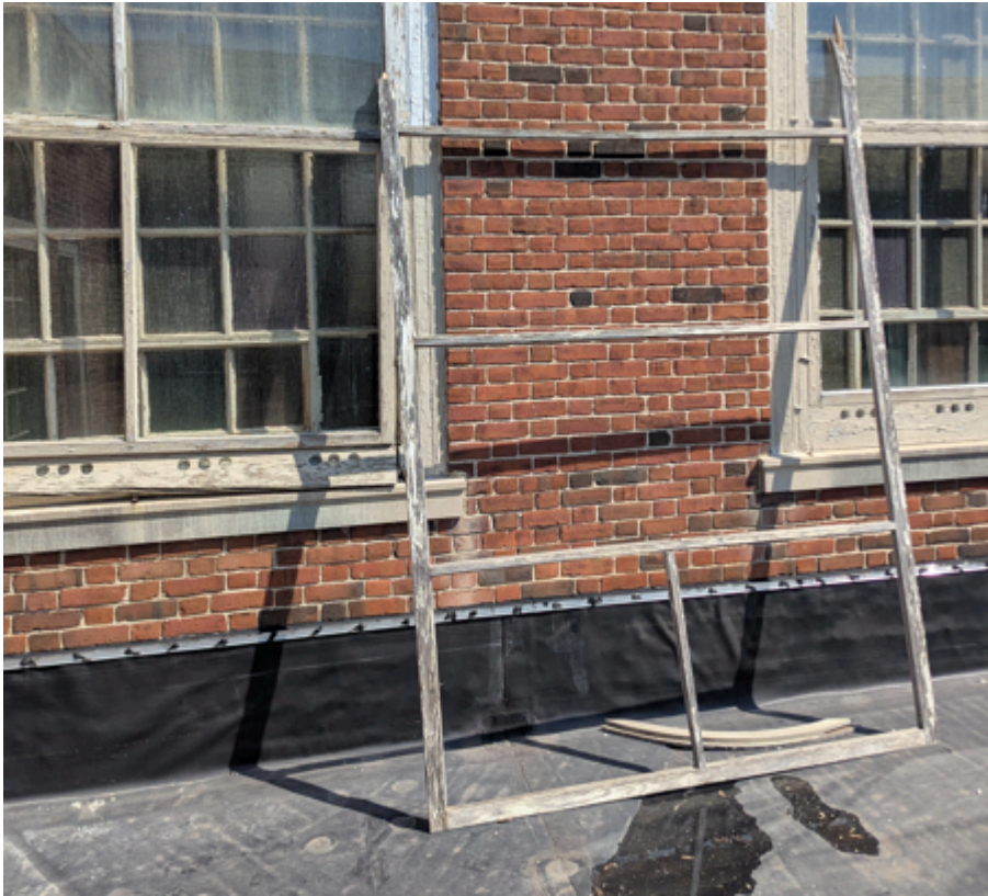
Destroyed Chapel Storm Window
