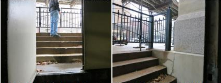
Stair 8 from the inside looking out. The exterior stair and railing will be demolished during the foundation repair work. Note the inadequate size of the exterior landing.
