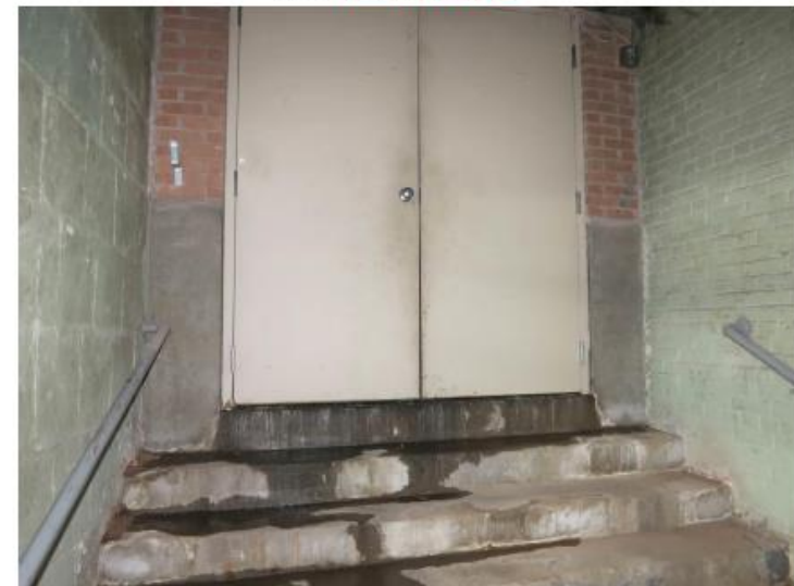
Exterior doors to Stair 8 from the inside. The poured concrete stair and surrounding construction seen here will be demolished in the foundation reconstruction. Stair does not meet current code. The pair of entrance doors swing into the space and a landing is required on both sides of the door.
