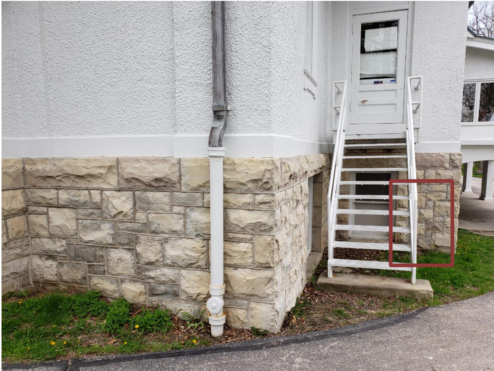
Image of the set of stairs under which the new condenser unit will be partially located, a rough estimation is indicated in red.
