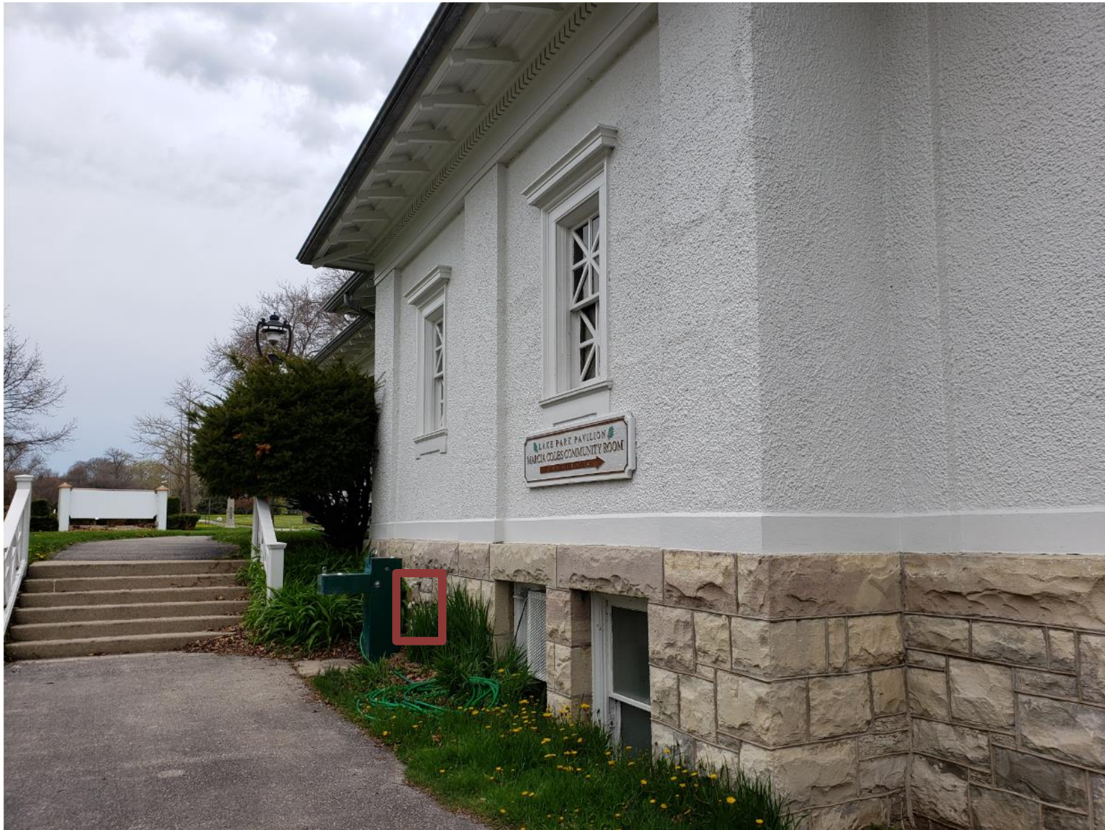
Image of the south elevation with an approximation of the location of the new air intake gooseneck (behind the drinking fountain) in red
