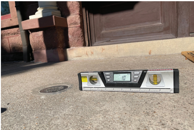
IMAGE 16: Concrete-porch floor slopes away from drain.
