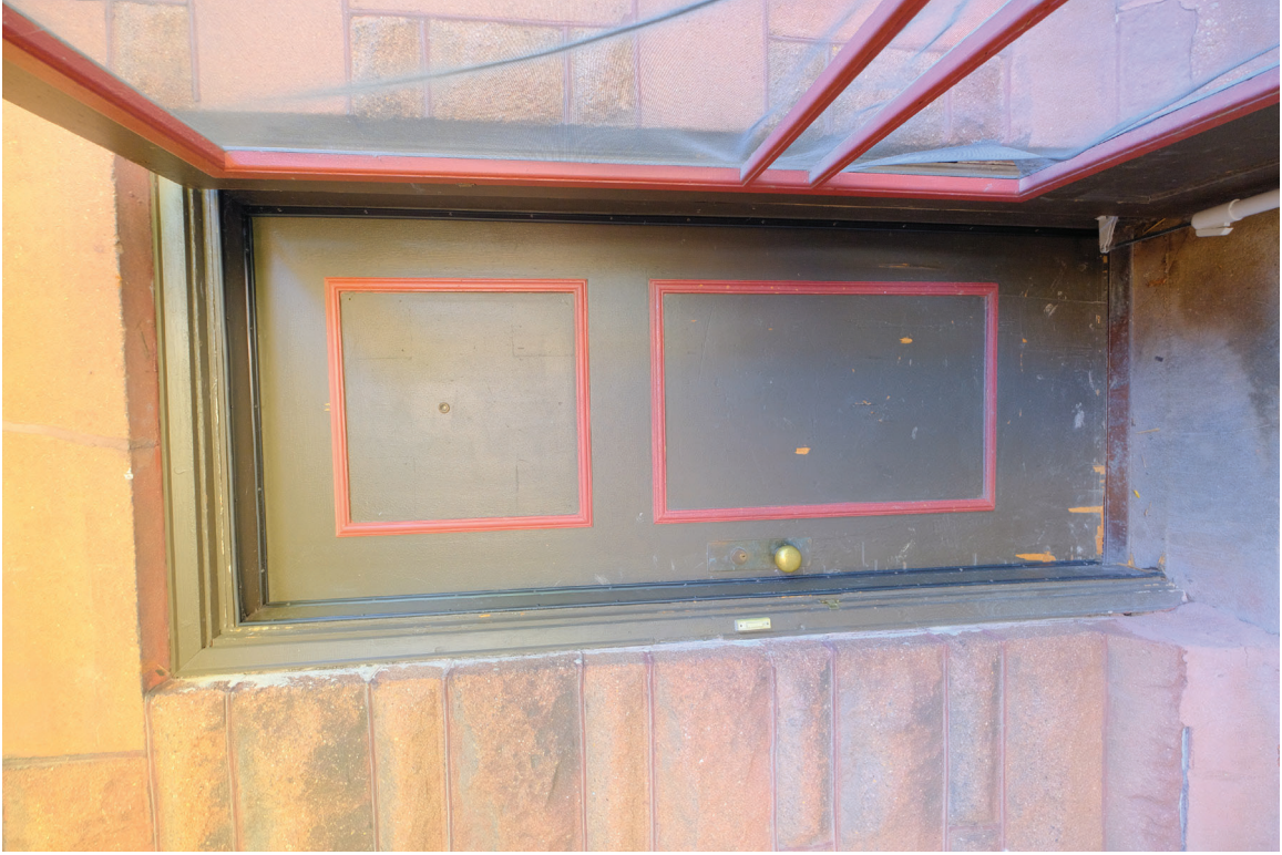
IMAGE 20: West entry door is in poor condition.
