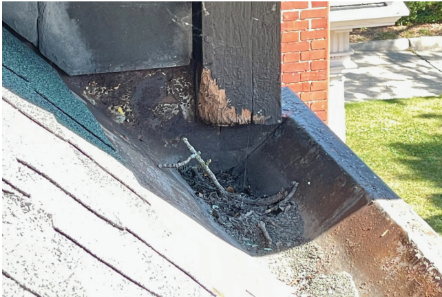
IMAGE 4: Debris and corrosion in built-in gutters.
