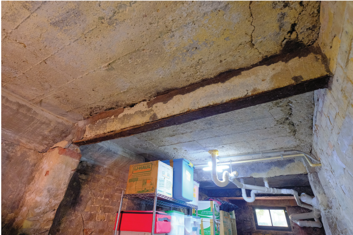
IMAGE 18: Cast-iron beams in the basement are severely corroded.
