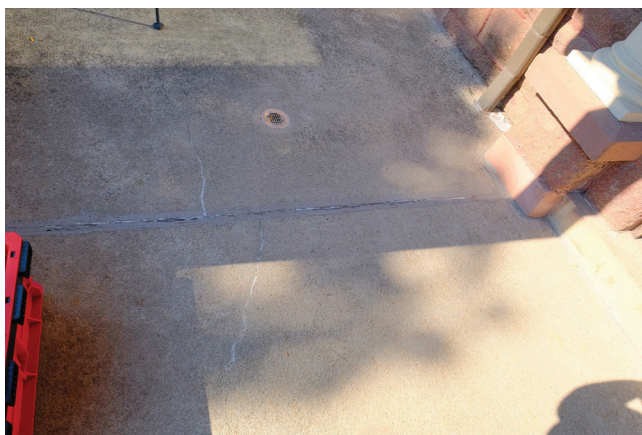
IMAGE 17: Cracking in the concrete-porch slab.
