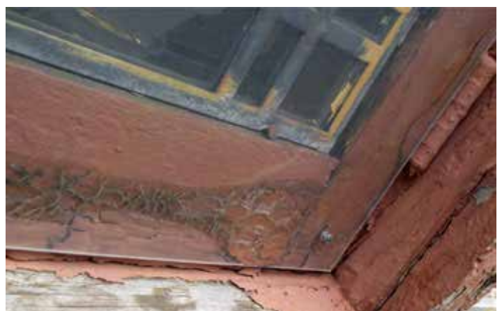
Lead paint chipping from a window.
