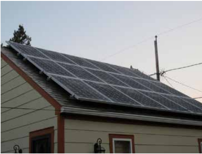
Example of rooftop solar.
