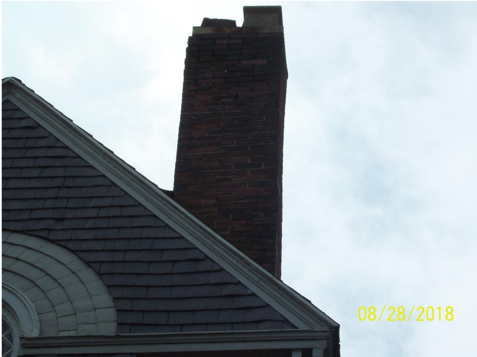
Inspector photo of chimney. Flue caps must be reproduced to match exactly.
