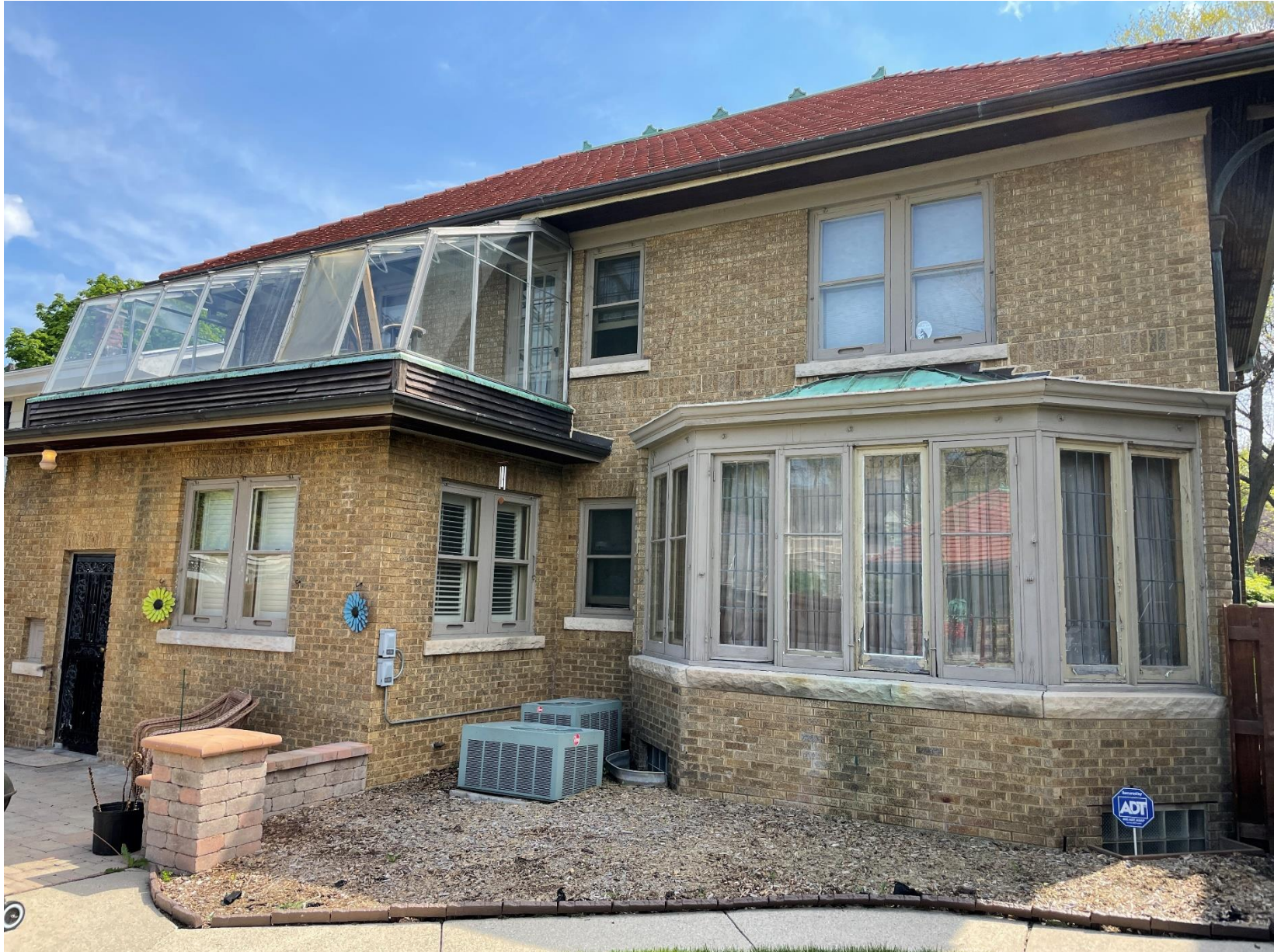
Storms to be replaced are primarily on the bay.
