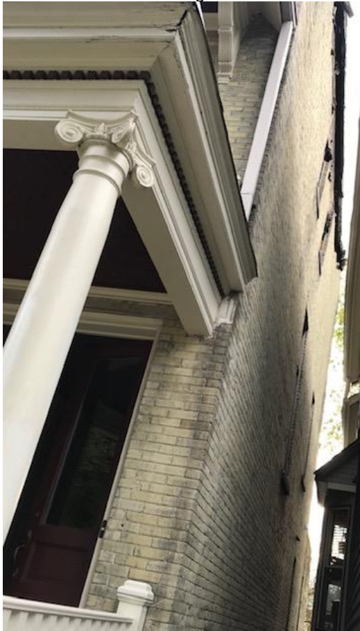
NE View Toward Damaged Wall
