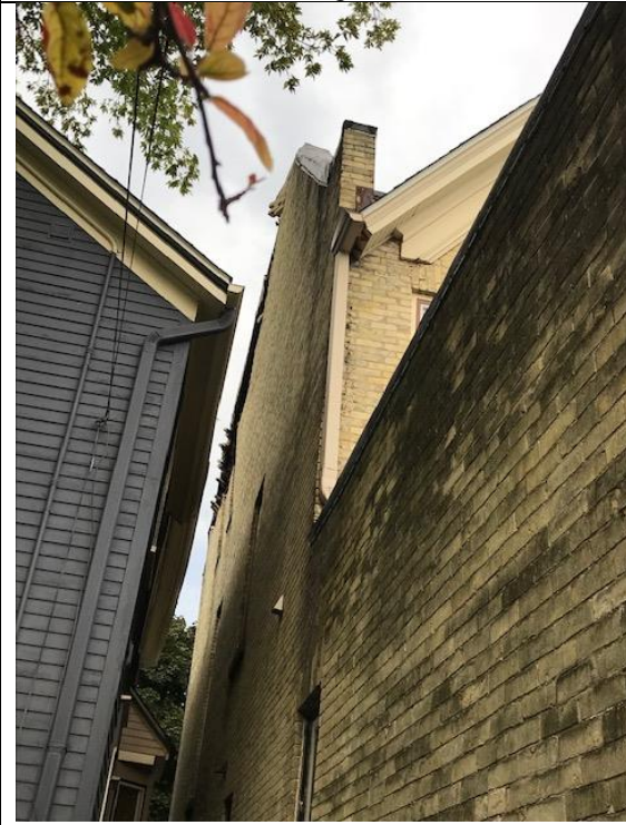
NW View Toward Damaged Wall
