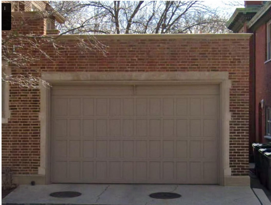
Area of coping stones to be treated with sealant, presumably to address efflorescence issue.
